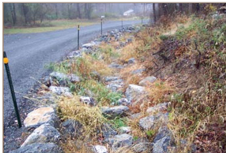
This conservation LID includes a driving surface aggregate, large stones to line the roadside ditch, new cross pipes and construction of plunge pools to slow down-hill, storm-water flow rate. Photo courtesy of the Iowa Natural Resources and Conservation Service, U.S. Department of Agriculture
