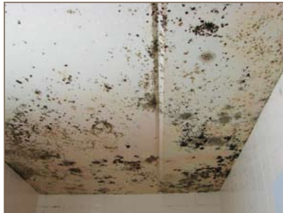
Mold growth on a bathroom ceiling is due to inoperable exhaust fans and inadequate dehumidification. Photo courtesy of Directorate of Public Works, Fort Polk
