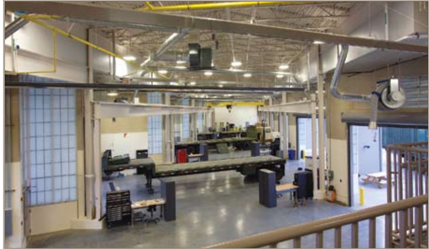
The NCARNG's field maintenance shop features a geothermal heating and cooling system, water-reducing facilities, occupancy-sensor lighting systems and tankless water heaters. U.S. Army photo
