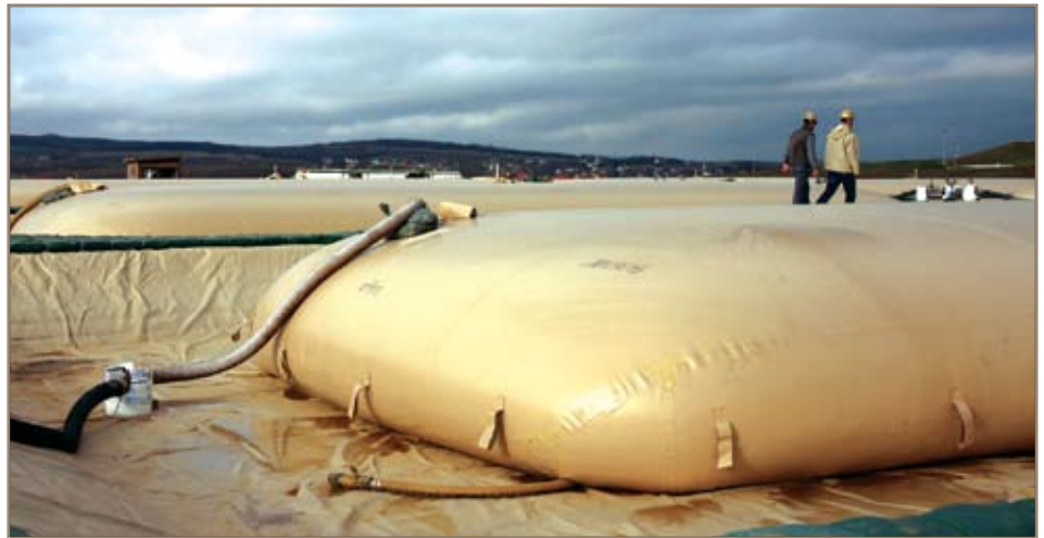
Kellogg, Brown and Root contractors walk by a 50,000-gallon bladder of diesel fuel on their way to install a unique manhole system that will provide secondary containment of any spill or contamination to the area. Photos by Justin Ward
