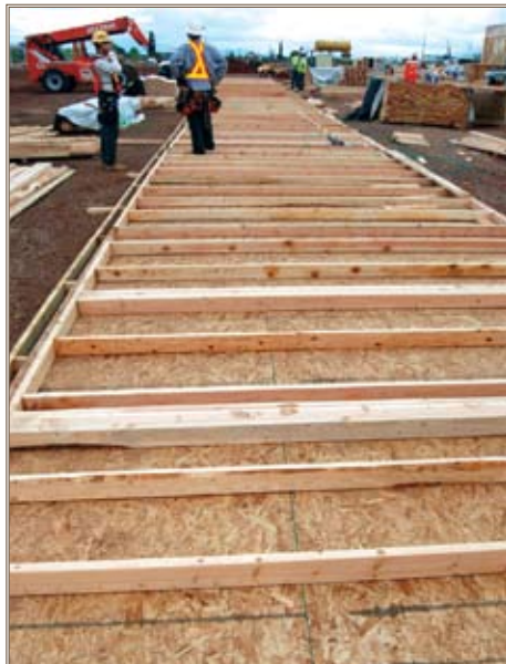
Contractors at a barracks under construction on Fort Huachuca inspect what will be a wall built using wood from suppliers certified by the Forestry Stewardship Council or who follow similar practices. Photo by Daniel J. Calderón
