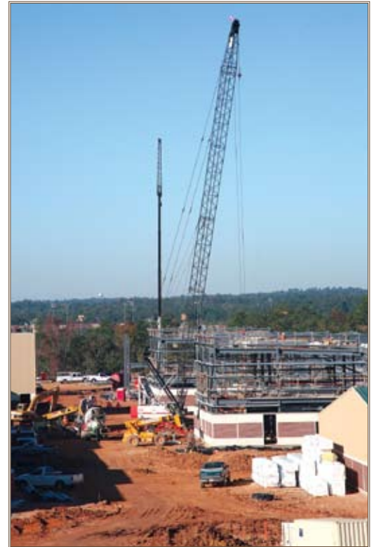
As contractors complete one phase of construction of barracks at Fort Benning, Ga., they repeat the process in the next. Photo by F.T. Eyre
