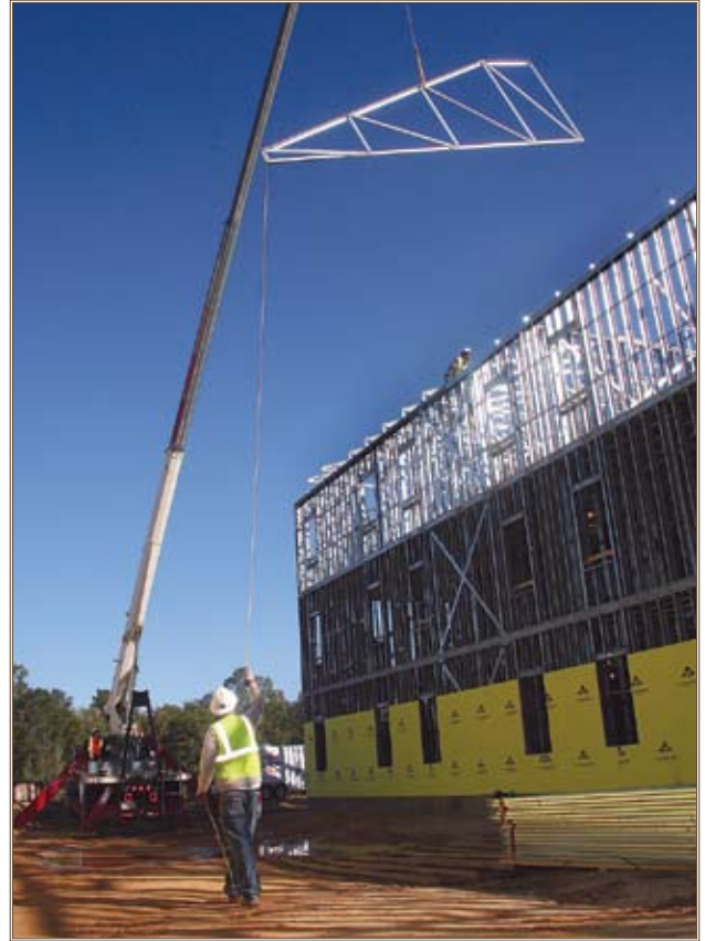
Workers use a construction crane to maneuver a roof element into place while building barracks at Fort Benning, Ga. Photo by F.T. Eyre
