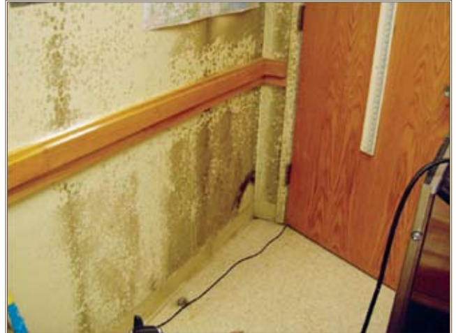
Before treatment, this barracks room wall is covered with mold. Photos courtesy of Pat Fields
