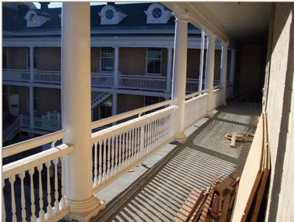
The modifications to Building 2000 include repairing or replacing wooden porch decking, railings and columns. Photos courtesy of JPMO
