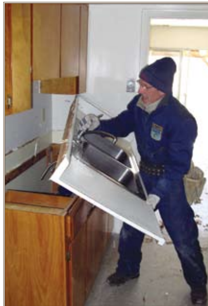
Habitat ReStore worker Darrell Cone removes a sink and countertop from a housing unit being deconstructed in Fort Leavenworth's Kickapoo Village. Photo by Will King.
