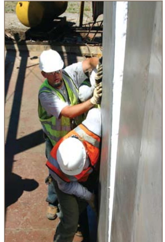
Workers build an insulated enclosure around the TNT washout facility equipment at Tooele Army Depot, Utah. Photo by Debra Valine
