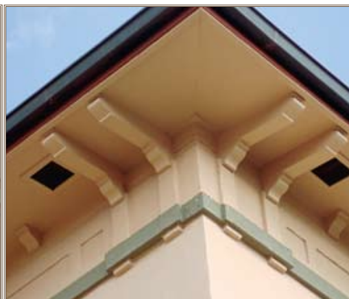
Over time, architectural features like these brackets were knocked off of the quads. The renovation team made plaster casts of surviving brackets in order to recreate and replace missing brackets. Photo by Ken Hays
