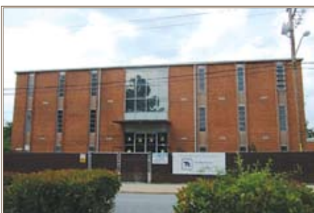
This 40-year-old Advanced Individual Training barracks at Fort Gordon, Ga., is being renovated to provide standard quarters for Soldiers and extend useful building life. Photo and rendering courtesy of U.S. Army Corps of Engineers, Savannah District
