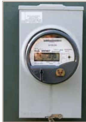
A TWACS meter for a 600-amp, 480-volt service is installed on the cooling system at Building 2878. Photos by Michael Aident
