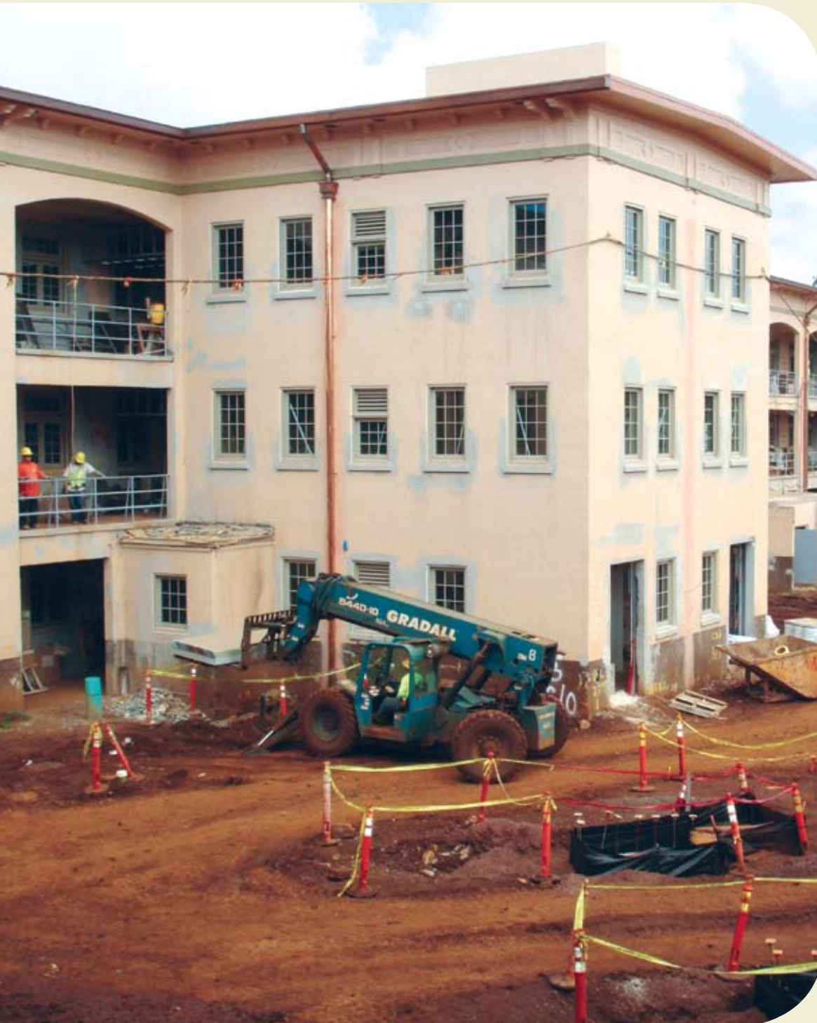
Construction at Quad E is part of the Whole Barracks Renewal Program at Schofield Barracks, Hawaii. Photo by Ken Hays. Page 10
