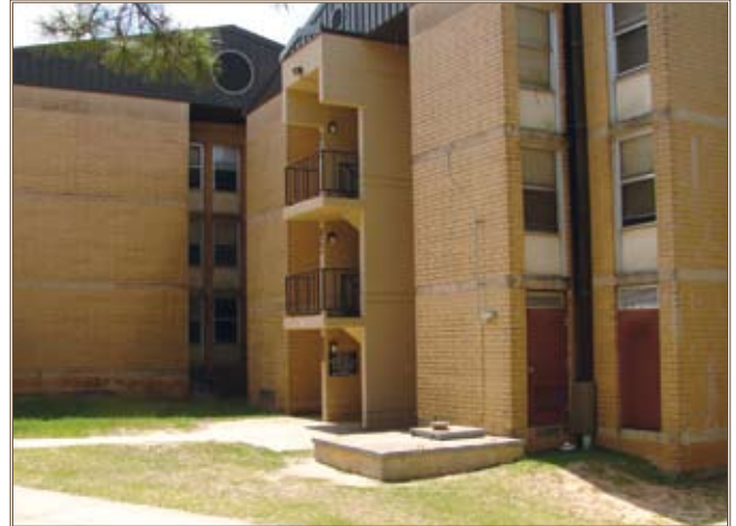
This 1970s barracks at Fort Polk, La., exhibits the mold and mildew problems common to similar structures in wet climates. Photos courtesy of U.S. Army Corps of Engineers, Fort Worth District
