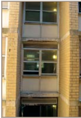
Condensation causes damage like that evident on this barracks at Fort Polk, La.
