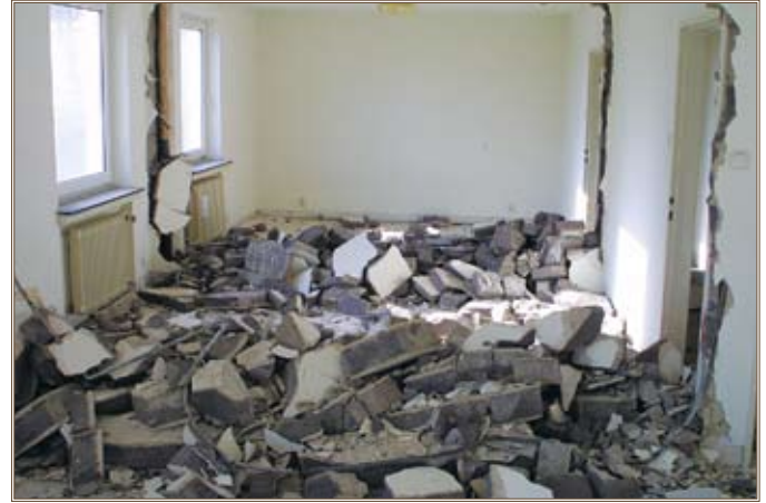
Rubble from the interior walls of an apartment in the Aukamm neighborhood covers the floor during an early stage of renovations.
