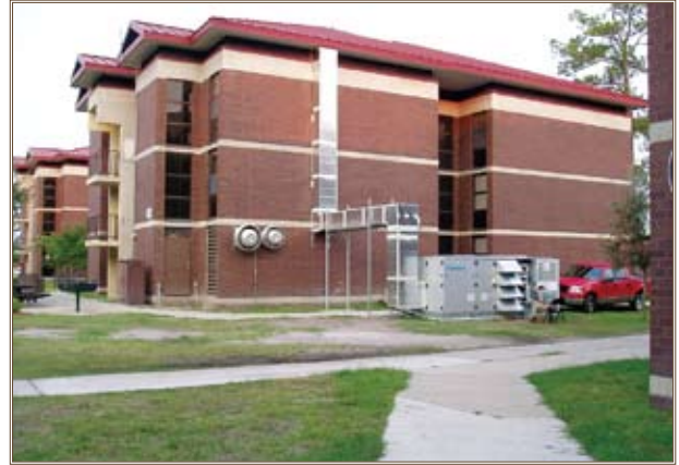
One of the DOAS being tested at Fort Stewart, Ga., uses a commercial off-the-shelf system to precool and pre-dry the outdoor air. Photo courtesy of ERDC-CERL
