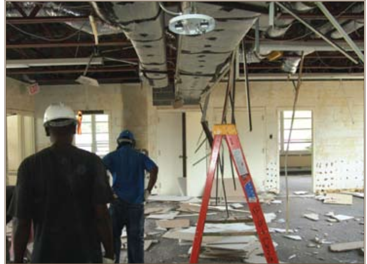
Crews demolish all building systems and finishes down to bare structure to enable renovation to modern systems, layout and finishes. Photos by Hillary Torchia, U.S. Army Corps of Engineers, Savannah District
