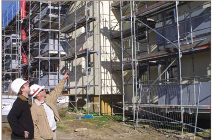
Michael Dennis, the Corps' senior construction control representative for Wiesbaden Family housing renovations, explains the scope of effort to a construction crew member. Photos by Evan Duncan
