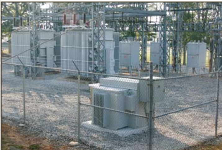
The control system communication equipment (foreground) sits inside the Mannfield electrical substation fence.
