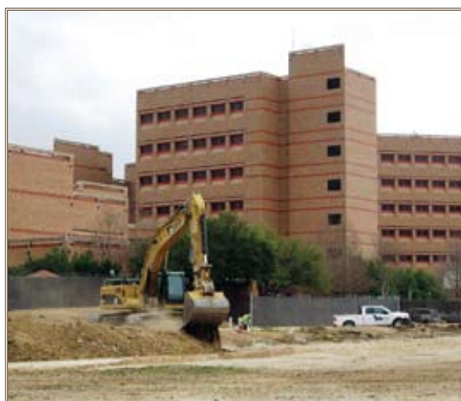
The Joint Center of Excellence for Battlefield Health and Trauma Research is under construction adjacent to Brooke Army Medical Center. Photo by Brian Dwyer
