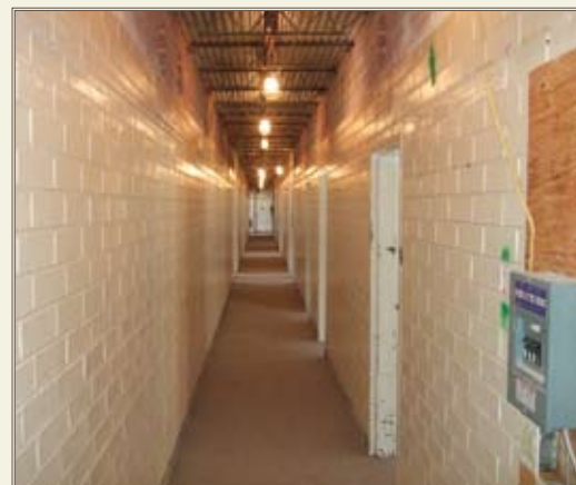
Existing narrow interior hallways will become utility corridors once exterior walkways are added.
