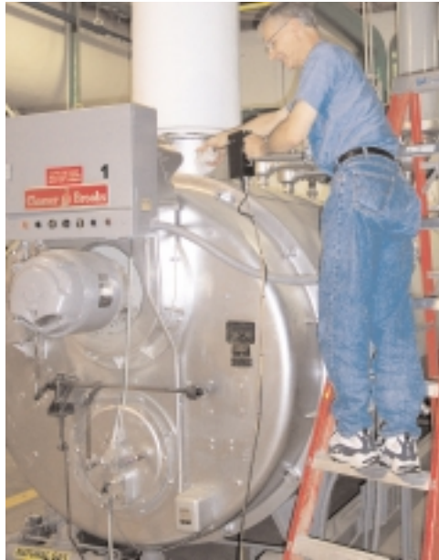
Noel Potts of the U.S. Army ERDC-CERL measures boiler stack gas emissions and boiler efficiency with a portable combustion analyzer.
