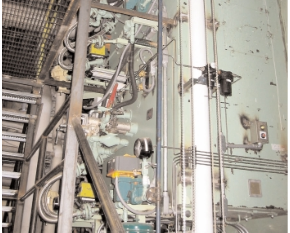
Front of the new Boiler #1 commissioned in 2003.
