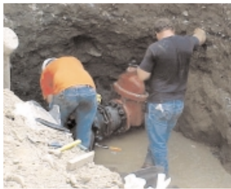
Old water main located on West Point reservation buried approximately 10 feet below the surface.
