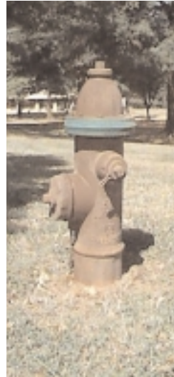
A fire hydrant that meets the Army standard.
