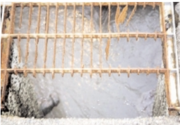
Corroded grating at wastewater treatment plant.
