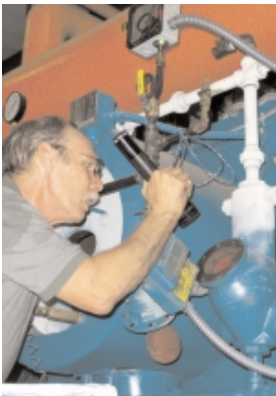
Boiler inspector examines the low water cut-off / control of water tube boiler at Fort Knox, KY.
