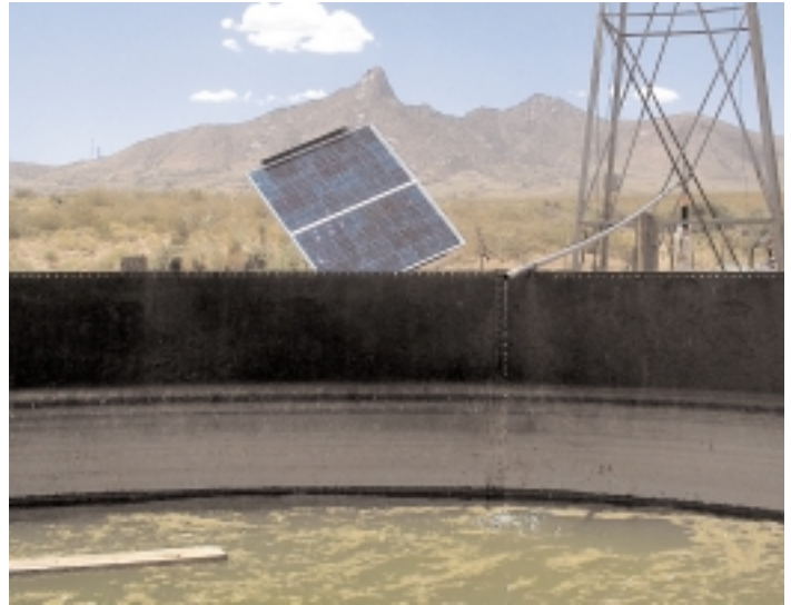
Solar-powered water well at Lena Cox Boone Ranch, White Sands Missile Range, New Mexico.
