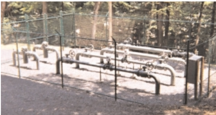
The new "Crow's Nest" natural gas regulator station.
