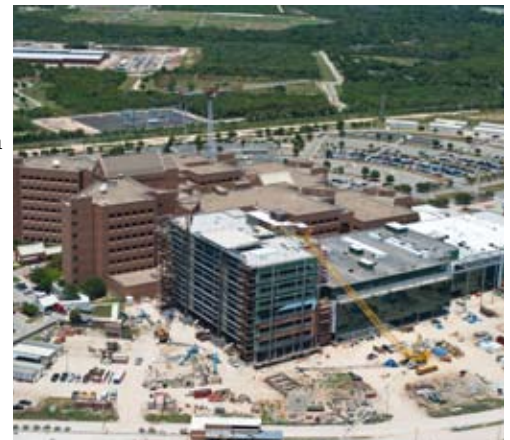
A seven-story addition is being built next to Brooke Army Medical Center.
