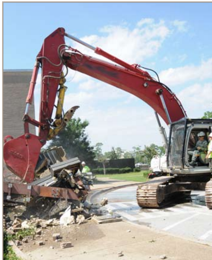
Air Force Brig. Gen. Ian Dickinson, 81st Training Wing commander, uses an excavator to begin demolition of a lodging facility at Keesler Air Force Base, Miss., one of three buildings being demolished there under an IDIQ task order issued by Huntsville Center's FRP. Photo by Kemberly Groue, U.S. Air Force
