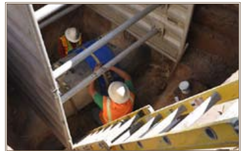
A Los Angeles District project is replacing 1940s-era steel and concrete water pipes with HDPE pipe at Vandenberg Air Force Base. Photos by Elizabeth Casebeer
