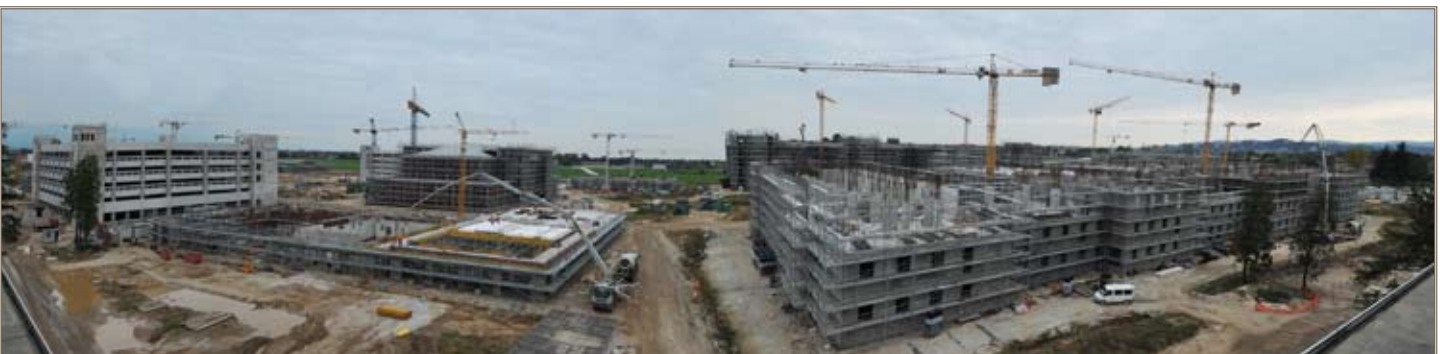
Construction progress is more than 30 percent complete at the Dal Molin site, future home of the 173rd Airborne Combat Team. Photo courtesy of the Naval Facilities Engineering Command, Vicenza, Italy
