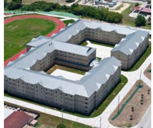
One of three dormitories on the Medical Education and Training Campus, which is geared to attain LEED Silver certification, is under construction.
