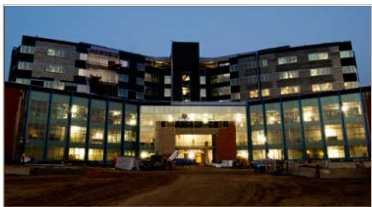
The Fort Belvoir, Va., Community Hospital, being constructed by USACE’s Norfolk District, will have a number of green features, including a roof designed to collect rainwater that will be used to irrigate the hospital grounds. Photo by Marc Barnes
