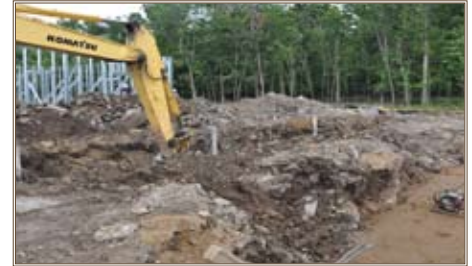
Crews work on trenches for geothermal wells at the Child Development Center under construction at Fort Drum. Photo by Dan Desmet, New York District
