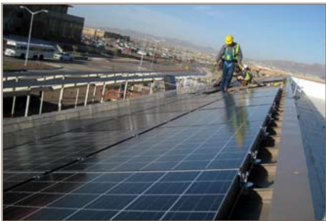
Workers install solar panels on the roof of a dining facility at Fort Bliss, an alternative energy program managed by Huntsville Center's UMCS program. Photo courtesy of Huntsville Center
