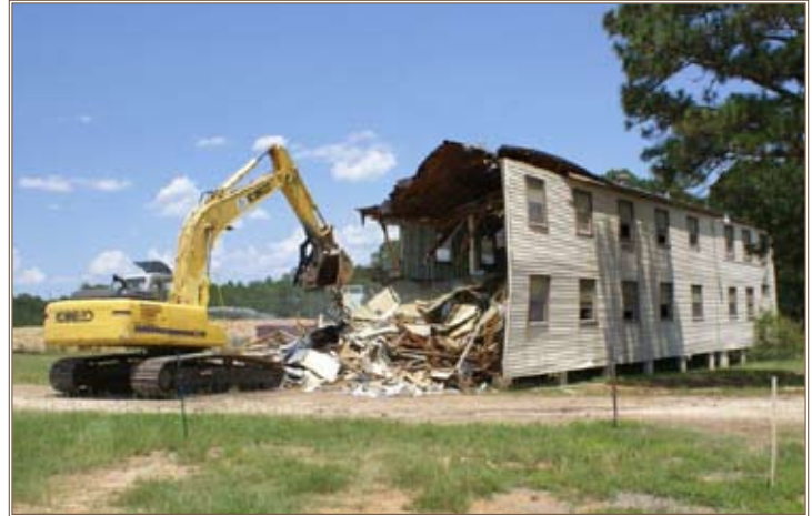
A backhoe takes down a 4,830-square-foot building, one of two structures at Fort Polk, La., demolished in 60 days by Huntsville Center's Facilities Reduction Program. Photo courtesy of Huntsville Center
