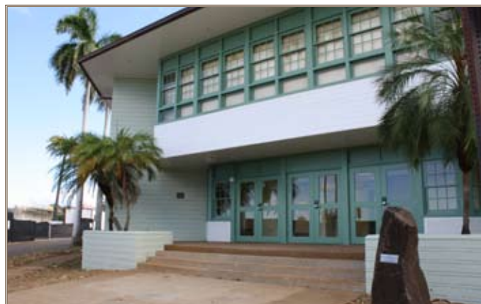
Fort Shafter’s Aloha Center entrance, following the recent rehabilitation project, matches the original from the 1940s. Photo by Dino W. Buchanan
