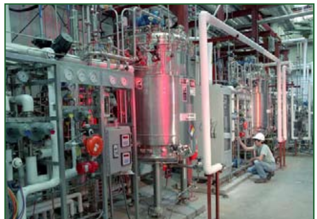
Facility and utility managers should understand where potential utility reliability issues of the infrastructure for which they are responsible exist. Photo by David Parsons
