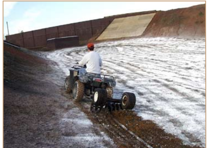
Engineer Research and Development Center researcher Jared Johnson applies lime in a grenade bay. Photo by Andy Martin, Environmental Laboratory, Engineer Research and Development Center
