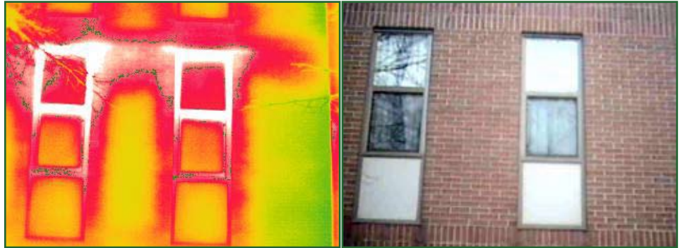
Thermographic image (left) of retrofitted barracks' windows (right) shows energy leakage. Photo by Alexander Zhivov, Construction Engineering Research Laboratory, Engineer Research and Development Center
