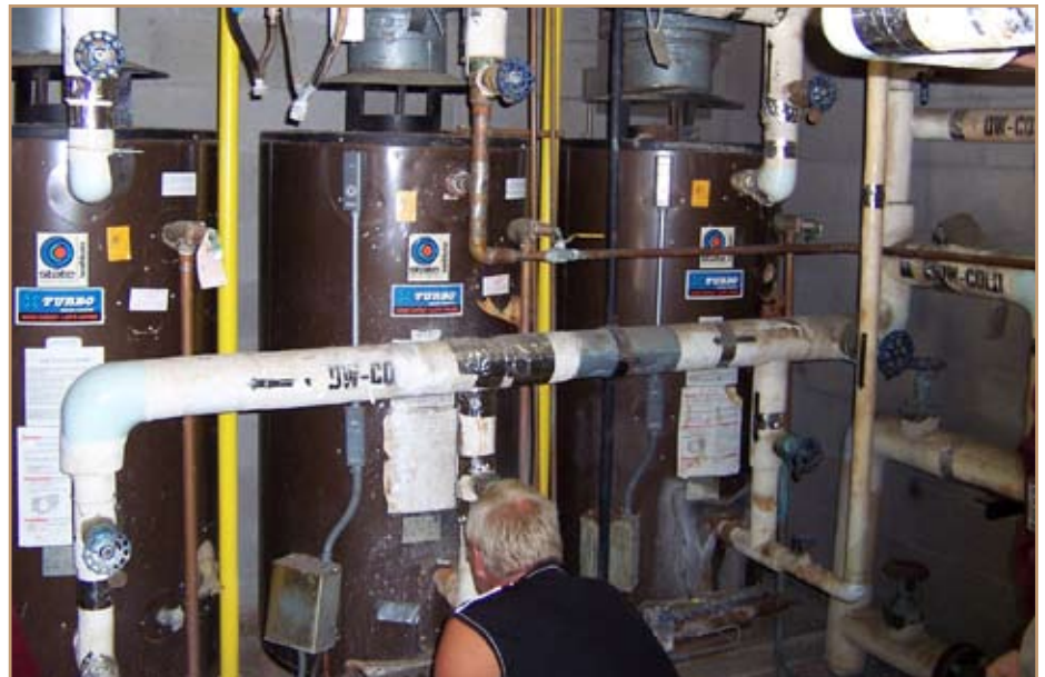
An engineer checks the temperature setpoint of domestic hot water heaters. Photos by David Underwood, Construction Engineering Research Lab, U.S. Army Corps of Engineers
