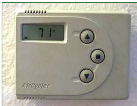
Turning off heating and cooling systems when the outdoor temperatures are in the low- to mid-70s is one way to reduce energy use.
