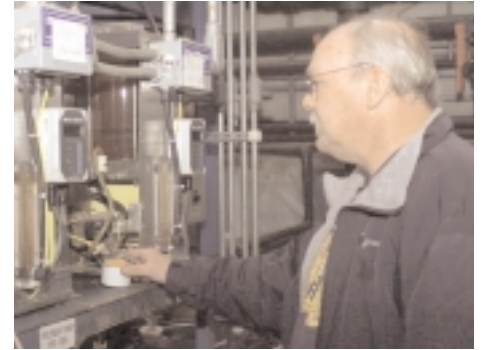
Wayne Jones, wastewater treatment plant operator, adjusts the polymer pump at the depot's groundwater treatment plant used in Anniston installation restoration activities.
