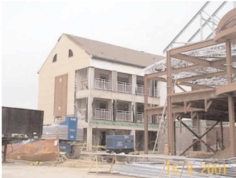
The barracks upgrade project at Fort Bragg involved removing the entire building to the concrete structure and rebuilding to improve living conditions and enhance soldier retention.
