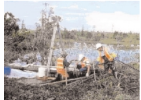
Manually draining a pipeline in a sensitive wetland environment, Annette Island. (Photo by Robert Gatewood, Summer 2000)
