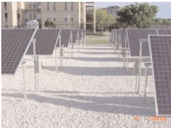
Each bank of photovoltaic panels is individually fused. Eight panels connected in a series deliver up to 400 volts DC.
