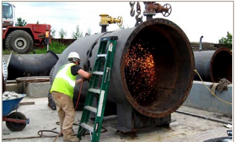
The St. Bernard Parish Pump Station Rehabilitation project in New Orleans received a Design Excellence Award for Rehabilitation/Renovation/Restoration Project.
