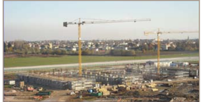
Two of the 22 cranes at Dal Molin support construction at two barracks that will house about 1,200 Soldiers. Photo courtesy of U.S. Army Garrison, Vicenza
