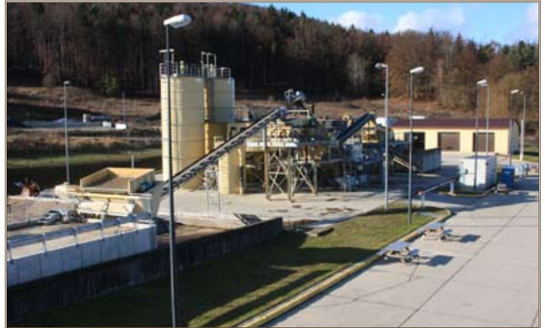
An additional external charging bunker with a grinding unit was installed to allow feeding of POL-contaminated soils into the treatment process at the wash rack at Camp Albertshof, Germany. Photo by Jochen Doerr
