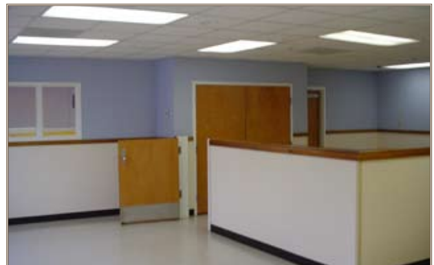
After the renovation, the lower four feet of the classroom walls are covered with vinyl wallpaper and capped with a chair rail.
