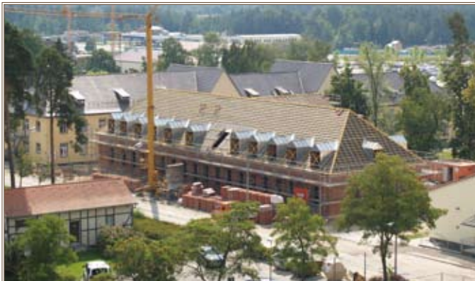
A battalion headquarters building is under renovation at USAG Grafenwoehr, part of EB-G.
