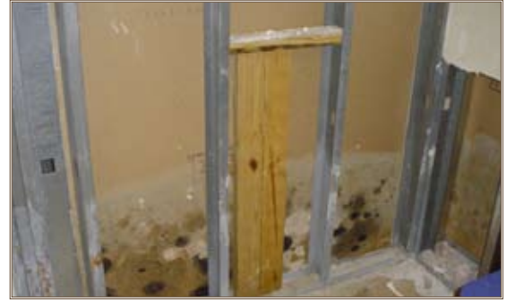
Before the renovation, mold grows inside an interior wall in the Santa Fe CDC at Fort Benning, Ga. Photos by David Miller
