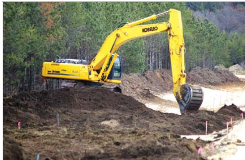
Employees from Fowler and Hammer Inc., of La Crosse, Wis., begin groundwork to construct a lane of the IED-Defeat Complex at Fort McCoy. Photo by Rob Schuette
