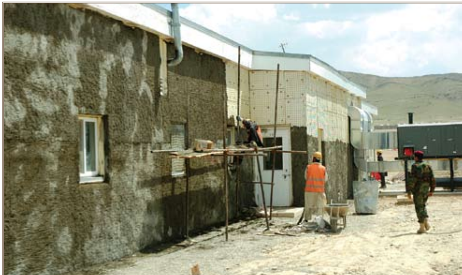
An ANA facility in Kabul, Afghanistan, undergoes renovation work. Photos by Bruce Huffman, AED Public Affairs
