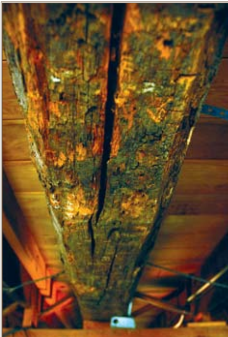
Floor joists, viewed from the Rookery’s basement, are estimated to be about 180 years old.
