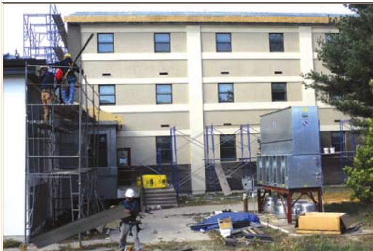
Construction workers labor on the AIT barracks project at Fort Meade, Md. Photo by Pfc. Ali Hargis
