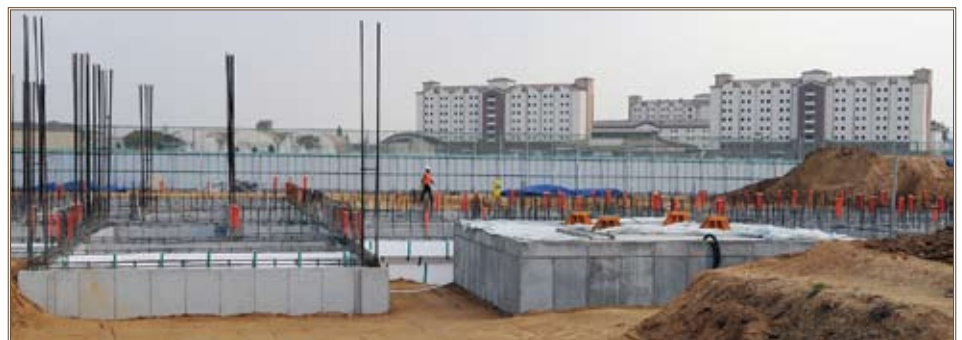
Construction of six single-Soldier barracks is underway on Parcel One, the newest land added to USAG Humphreys. In the distance are two new Soldier barracks and a dining facility.
