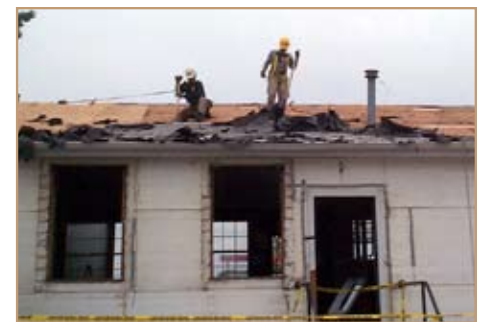
Workers remove asphalt shingles during a pilot deconstruction project at Fort Campbell, Ky., in 2002. Photo by Stephen Cospers
