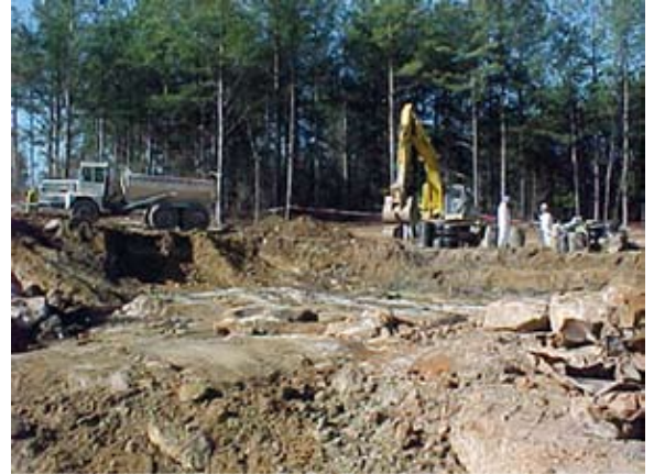
About 4,000 tons of soil contaminated with volatile organic compounds is removed from Fort Gillem, Ga., during an interim remedial action in 2001. Photo courtesy of Fort McPherson Public Affairs
