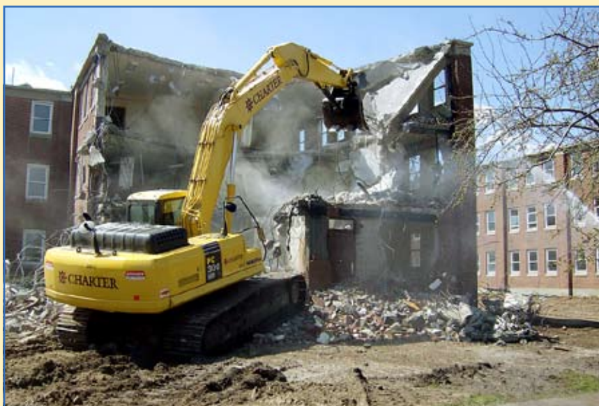
Charter Environmental begins the second phase of demolition of Building 408 at Fort Hamilton, N.Y., April 2. Phase one involved removing asbestos. The Engineering and Support Center, Huntsville's Facilities Reduction Program is working with the installation, the U.S. Army Corps of Engineers New York District and contractor partners to remove, by traditional demolition, three multi-use buildings that were employed as barracks, administrative and dining facilities. The plan is to recycle or re-use as much of the material as possible. Photo by Kevin J. Merenda, U.S. Army Corps of Engineers, New York District
