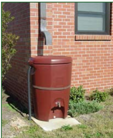
Rain barrels capture water for reuse at Fort Bragg, N.C.
