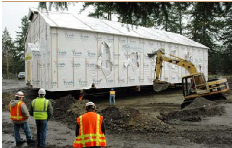
Rich Littooy, Barry Poirrer and Elizabeth Chien observe as the chapel is carefully placed at its new location. Littooy and Chien are with the U.S. Army Corps of Engineers, Seattle District, and Poirrer is the MCS Environmental superintendent. Photo by Kayla Overton
