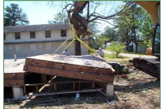
Mechanical equipment can make deconstruction more efficient. Here, a trackhoe lifts a section of floor structure during a demonstration project at Fort McClellan, Ala., in 2003. Photo by Joyce Baird
