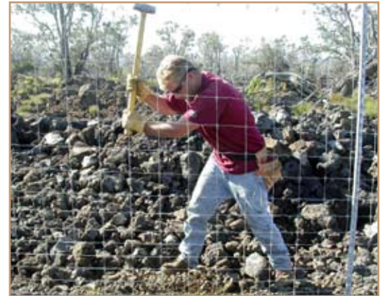
Contractor Tony Rosa pounds a stake into the ground to anchor a fence bottom at Pohakuloa Training Area. Once completed, about 70 miles of fence will protect threatened and endangered plants from goats, sheep and pigs. Photo courtesy of U.S. Army Garrison Hawaii Natural Resources
