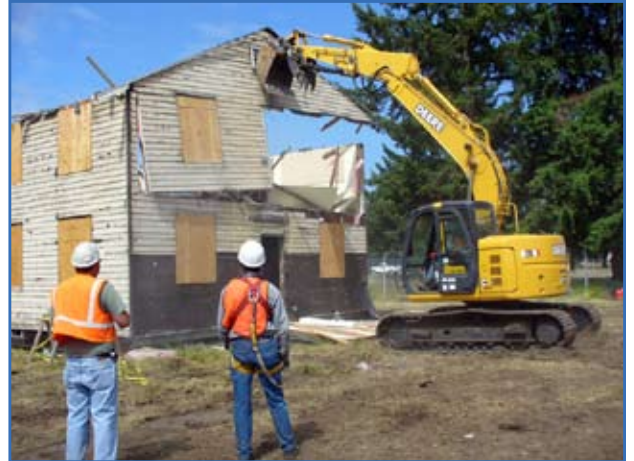
One of many World War II-era buildings at Fort Lewis, Wash., is "deconstructed" to increase the recovery of usable materials as well as the solid waste diversion rate of construction debris. Photo courtesy of Terry Austin.
