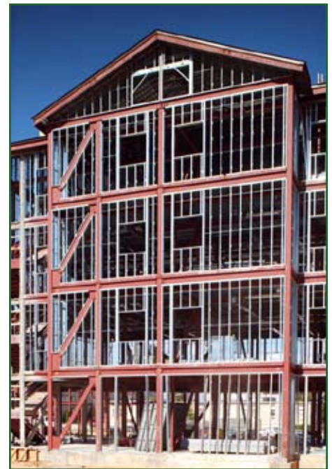
As in this barracks building at Fort Bragg, N.C., almost all steel used in new construction in U.S. Army Corps of Engineers’ Savannah District projects comes from recycled material. Photo by Jonas Jordan, Savannah District
