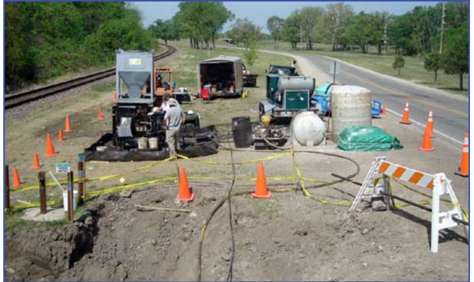
Workers drill under Union Pacific Railroad's tracks to place a cleanup project's injection equipment where it would not impact the endangered bald eagle habitat nearby. Photo courtesy of Herbert J. Abel
