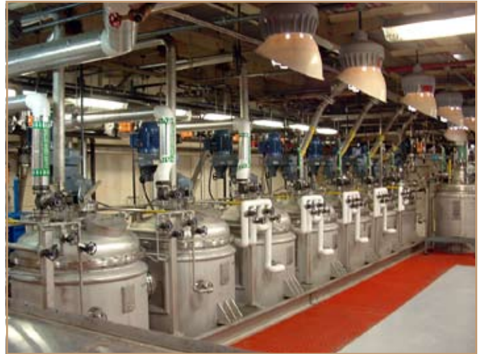
TNT weak nitric acid crystallizer vessels eliminate the generation of hazardous red water at Radford Army Ammunition Plant, Va. Photo courtesy of Brad Jennings
