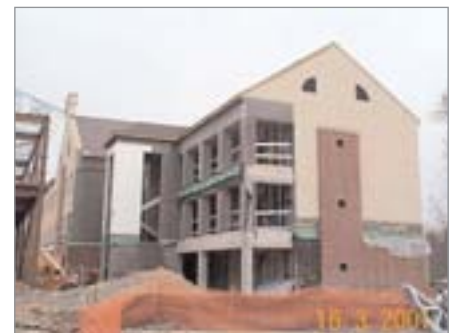
Remodeling jobs range from sprucing up a kitchen to total gutting, like this barracks at Fort Bragg.
