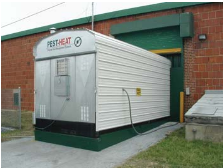
Thermal pest management chamber at Defense Distribution Depot Susquehanna, Pennsylvania.
