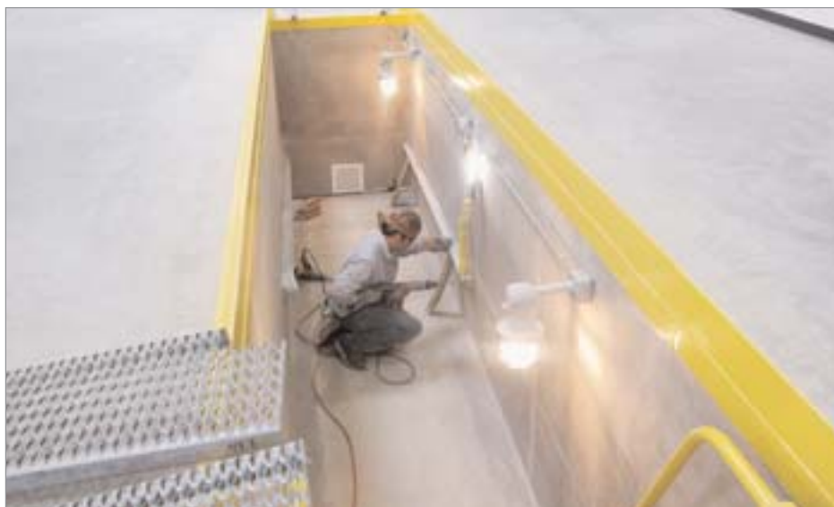
A subcontractor installs support for inspection pit grating at the transportation inspection point.
