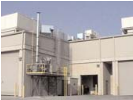
A catalytic Recuperative Thermal Oxidizer removes 95% of the VOCs and HAPs before discharging the exhaust air.
