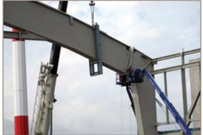
A structural steel installer at the $22 million Ramstein Air Base C-130 hangar bolts together sections of the 355-foot main beam. Photo by James Wofford, Europe District project engineer
