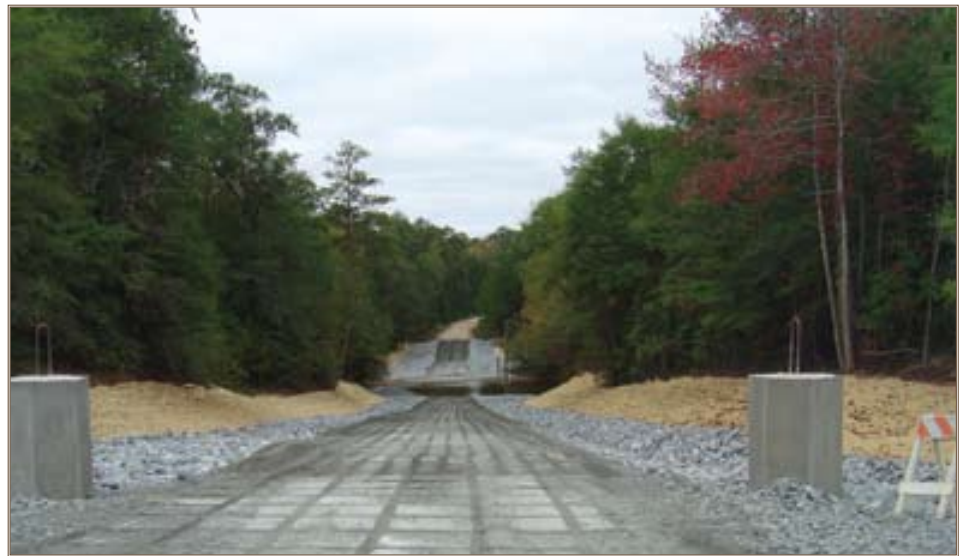
The low-water crossing sites were remediated with articulated concrete slabs, constructed with cable concrete, which allows for movement of the track vehicle. The cable concrete is placed underwater on the river bed to minimize the disturbance caused by the tank. Entrance and exit slopes are also hardened reducing suspended solids released into the waterway.
