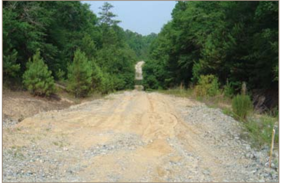
Remediation of three low-water crossings, like this one, was one of the projects that decreased environmental impact on training areas at Fort Benning. Photos by Johnny Markham, Fort Benning
