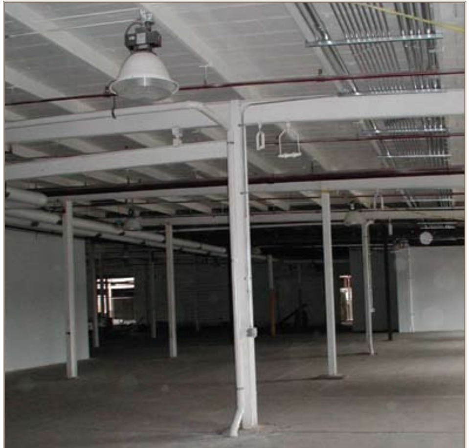
Pipes installed in floor slabs allow contaminated soil vapors to be drawn into a piping system and escape to the outside of a building. Photo by Mark J. Fisher
