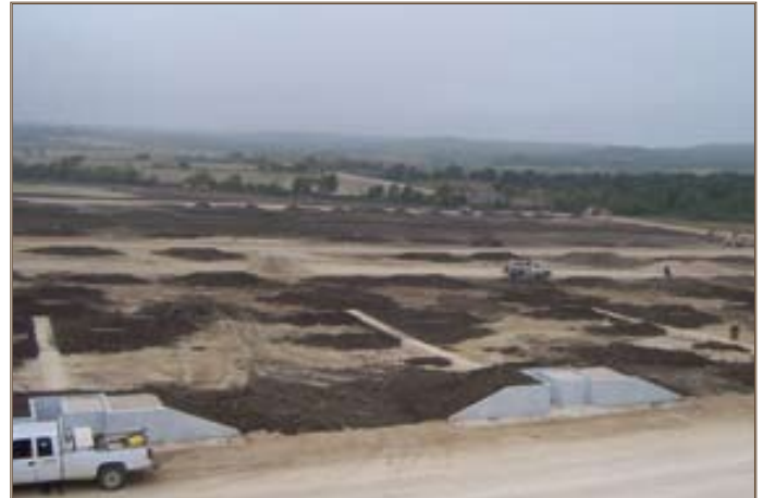
A state-of-the-art digital multi-purpose range, where Soldiers will be able to conduct gunnery training in a realistic environment, is under construction at Fort Hood. Photo by Michelle Lenis
