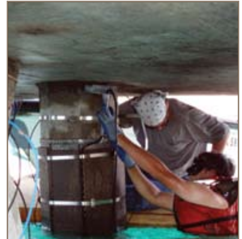
Divers install a composite wrap, a mesh material that provides cathodic protection, on dolphins at Kawaihae Harbor. Photo courtesy of CERL
