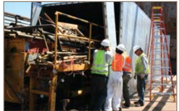
Workers build an insulated enclosure around TNT washout facility equipment at Tooele Army Depot, Utah. The FRP project employed, thermal convection to bring down an unwanted ammunition facility. Photo by Debra Valine
