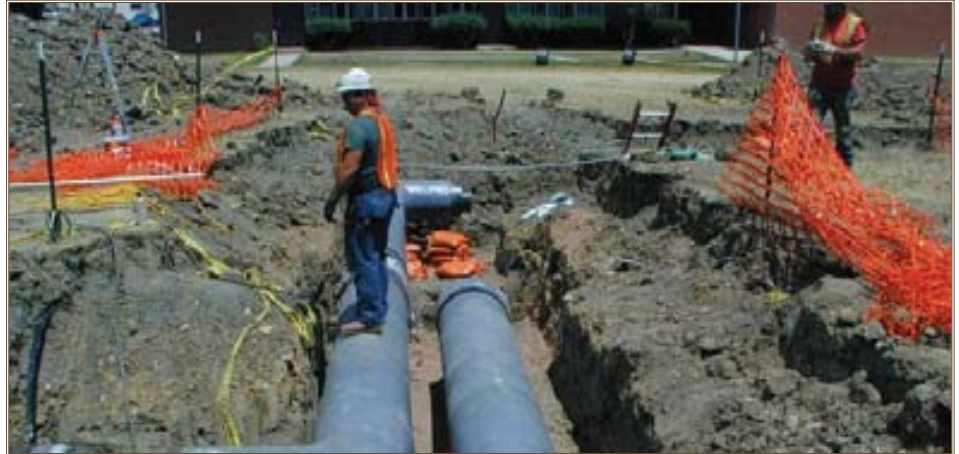
High-density polyurethane- and FRP-clad heat distribution pipes are being analyzed after three to four years in service. Photo courtesy of ERDC-CERL
