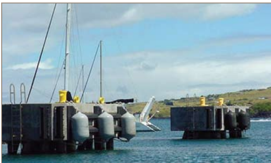
Dolphins in the Kawaihae Harbor are being used to study a composite wrap’s effectiveness in protecting against corrosion. Photo courtesy of USAG Hawaii
