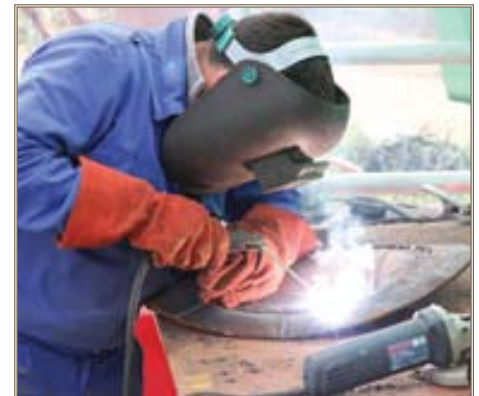
Sparks fly as a welder repairs damage to a water tower on Morón Air Base, Spain, where Europe District oversees the safety and quality of housing renovations and provides engineering and safety support on many other projects. Photo by Justin Ward
