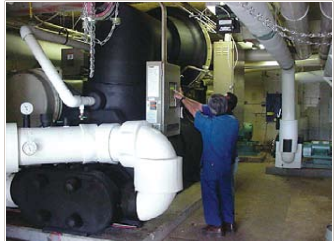
During retro-commissioning at USAG Hawaii, a chiller’s controls are examined. USAG Hawaii photo
