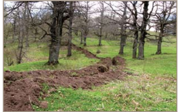
Water and sanitary lines near Sevkar, Armenia, are undergoing significant refurbishment, replacing old, rusted and disconnected waterlines and reservoirs with new pipes, fencing and connections, giving roughly 9,000 Armenians fresh water from their taps. Photo by Nana Kacheishvili, U.S. Army Corps of Engineers
