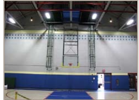
After energy-efficient lighting is installed, costs are reduced, and the gym is more brightly lit.
