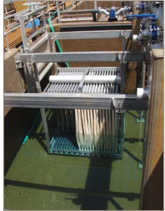
The Schofield Barracks Water Treatment Plant has been retrofitted with MBR systems that separate solids from water and wastewater. Photo courtesy of U.S. Army Garrison Hawaii
