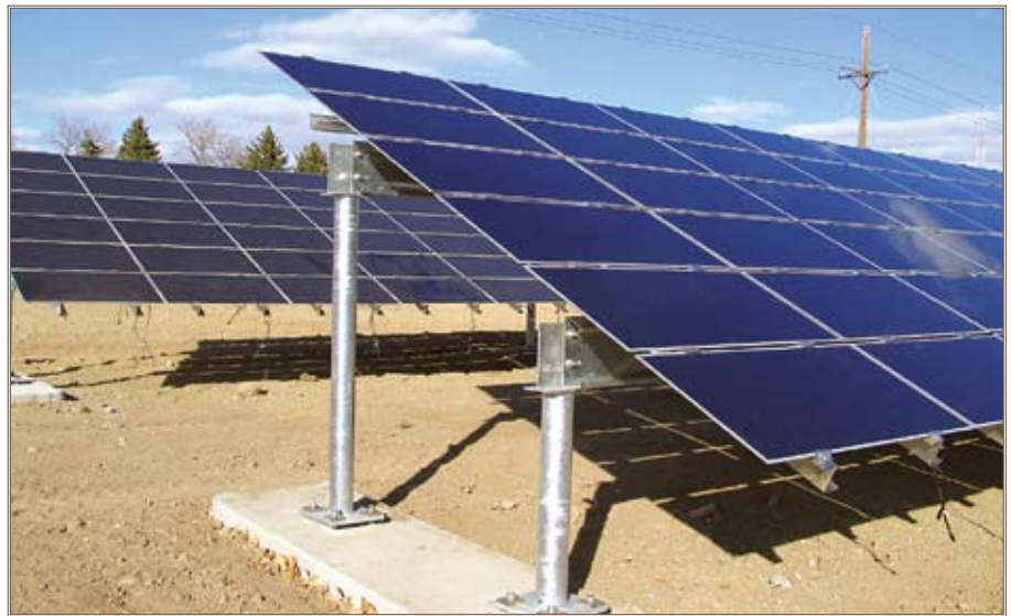
Solar arrays like this one at Fort Carson, Colo., reduce dependence on fossil fuels. Photo courtesy of ASA-I&E
