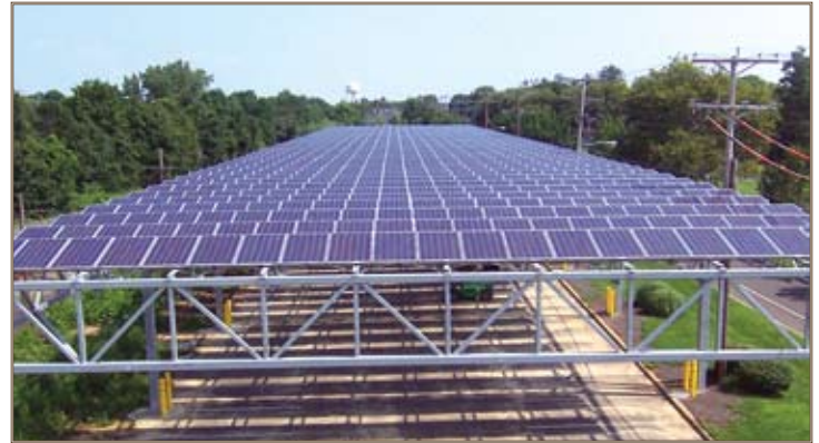
The New Jersey National Guard's photovoltaic system, built with ECIP funds at Sea Girt, N.J., produces 230 kilowatts of electricity. Photo courtesy of New Jersey National Guard
