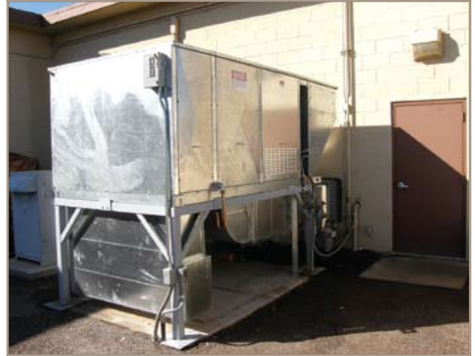
A 10-ton GHP is in operation at Luke Air Force Base, Ariz. Photo courtesy of ERDC
