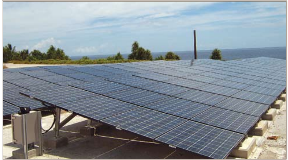
A solar electric system converts the sun's energy to electricity. Photo courtesy of Bill Stein
