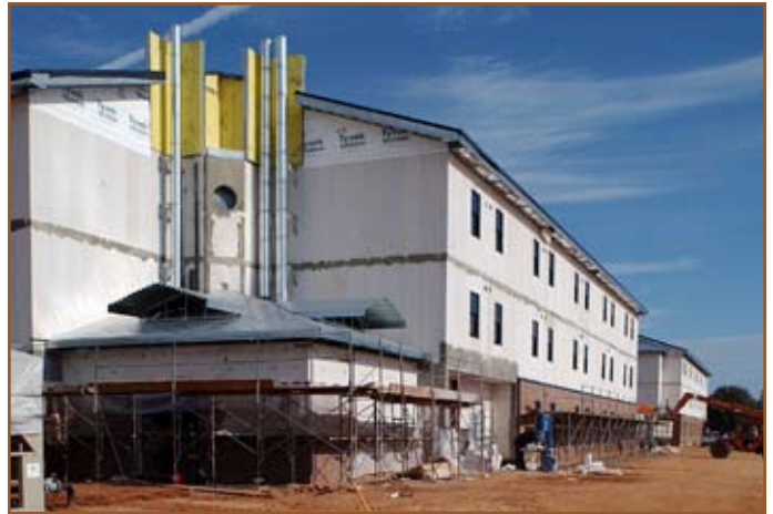
Relocation of the Armor School to Fort Benning, Ga., increases the demand for facilities like this barracks under construction. Photo by Jonas Jordan
