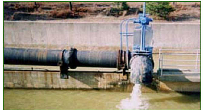
Innovative coating systems will be used to prevent further corrosion on an inlet pipe to a tank bath at Fort Bragg, N.C. Photo courtesy of the U.S. Army Engineer Research and Development Center
