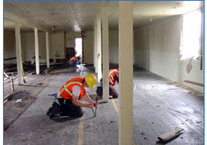
Contractors removing building materials from World War II barracks like this one on North Fort Lewis encounter lead-based paint contamination. Photo by Spc. Leah R. Burton
