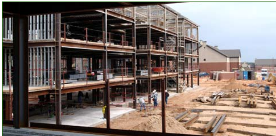
Work progresses on the 1st Brigade Barracks at Fort Bragg, N.C. Photo by Jonas Jordan
