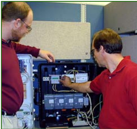
CERL's energy support is helping installations implement direct digital control systems with interoperability. Photo courtesy of the U.S. Army Engineer Research and Development Center
