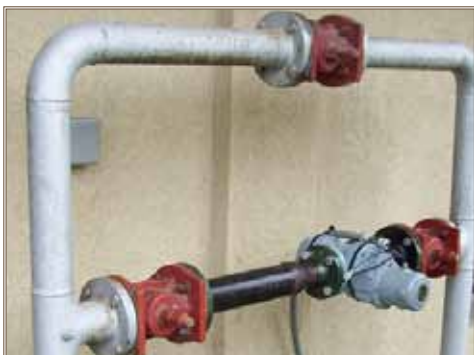
An advanced meter measures natural gas usage at Fort Hood, Texas. Photo courtesy of AMP
