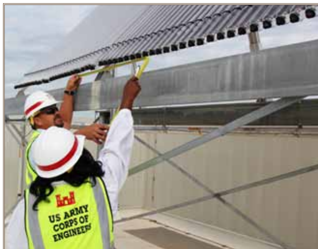
Tom Hordnes (top) and Patricia Smith, USACE construction inspectors, check the vacuum tube arrays of the solar panels that will save energy for Fort Jackson’s new Quad DFAC. Photo by Sean McBride, public affairs specialist, Charleston District
