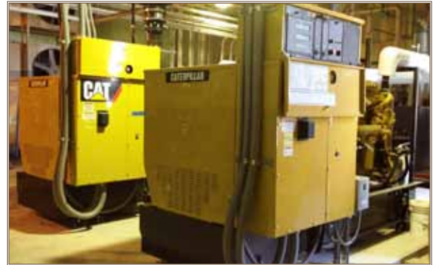
This emergency natural gas generator is part of the microgrid demonstration at Fort Sill. Photo by Misha Carlisle
