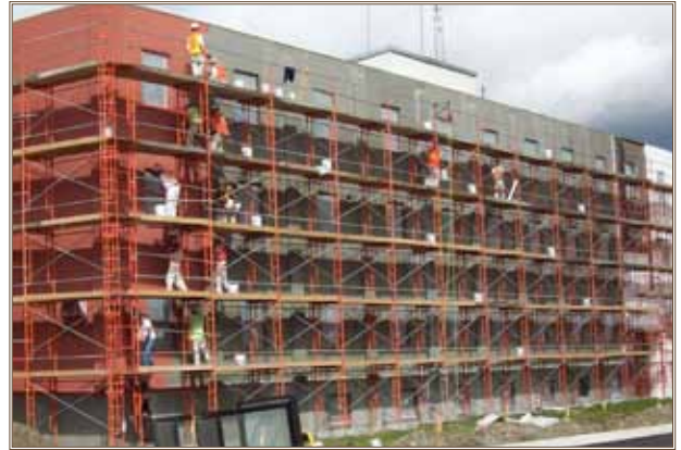
Workers install an external insulation finish system to improve the building’s energy efficiency at Fort Greely. Photo courtesy of DPW, Fort Greely
