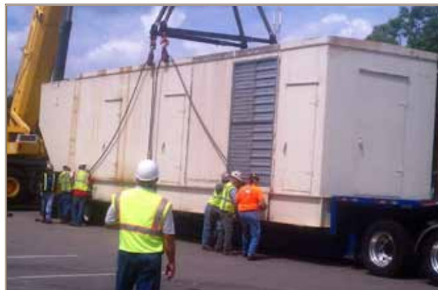
A Pentagon generator is offloaded after relocation to Fort Bragg as part of an energy security and peak-shaving project. Photo by Keith McAllister
