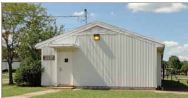
During assessments, inspectors look for easily fixable energy wasters like exterior lighting of buildings and grounds during daytime hours. Photos courtesy of Sain Engineering Associates
