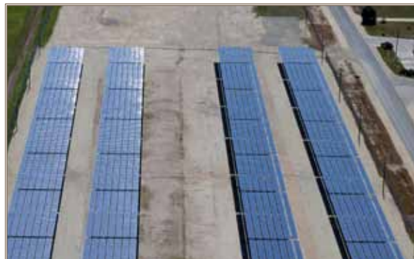
The IPT allows planners to evaluate building clusters to identify the right mix of different measures such as insulation, cogeneration, wind and solar power like this photovoltaic array at Fort Hunter Liggett, Calif. Photo courtesy of ERDC
