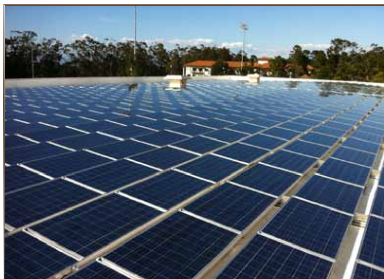
The Presidio of Monterey's Price Fitness Center rooftop solar array generates the power to make the center a net-zero electrical facility. Photo by Jay Tulley
