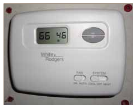
Improper heating and cooling thermostat set points are energy wasters noted by inspectors during assessments.
