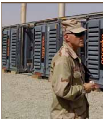
Hal Alguire checks out the leased internal combustion diesel generator plant at Camp Leatherneck. Photo by Ron Kaczmarek, director of Public Works, Joint Base Myer-Henderson Hall, Va.
