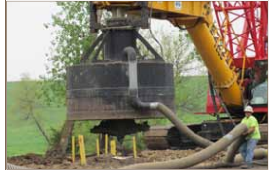
The large-diameter auger's bit is visible below the off-gas collection hood as a worker repositions the vapor collection line during treatment at the former Offutt Air Force Base. Photo by Charles Coyle
