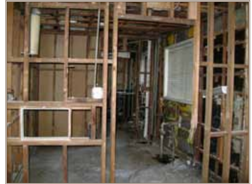
Structural and utility concerns behind the walls are uncovered during a USAG Yongsan renovation project. Photos by Bryan Dorrough.
