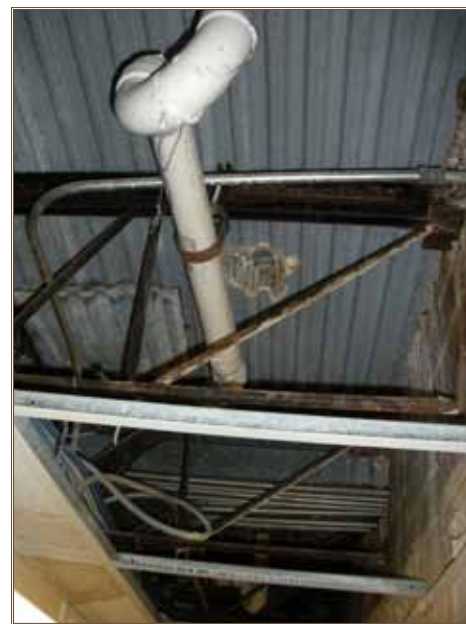
Removed ceiling panels exposes repairs that need to be done. Photo by Peter Thomas
