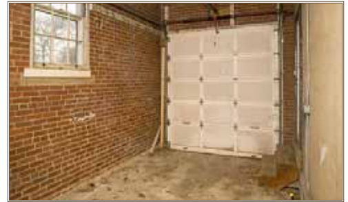
Before renovation, the garages in Fort Belvoir's Belvoir Village homes are narrow and unable to accommodate today's family vehicles. Photos courtesy of Fort Belvoir Residential Communities LLC
