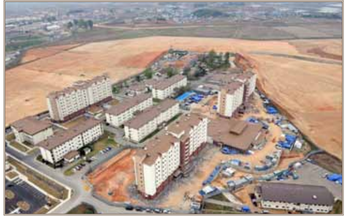
At Camp Humphreys, South Korea, permanent party barracks near completion. Photos courtesy of U.S. Army Corps of Engineers
