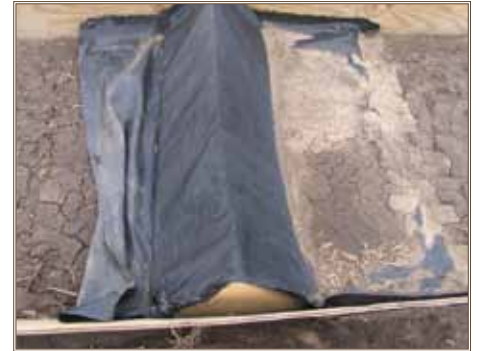
Sediment is captured by a triangular foam berm, a type of check dam commonly used on military lands that was evaluated. Photo courtesy of ERDC
