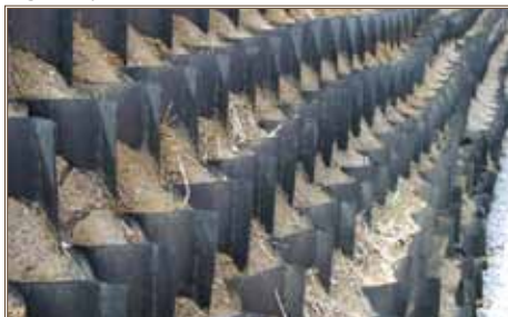
Camp Atterbury, Ind., is successfully using geogrid stabilization for some embankments. Photo courtesy of Engineer Research and Development Center
