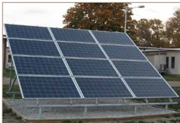
Photovoltaic array system at IAAAP is already capturing solar energy to create electricity for the building, and future projects may expand its use.
