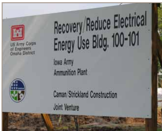
Contractor-Project Identification Sign: Sign at IAAAP announces construction of new geothermal and photovoltaic systems at its administration building.
