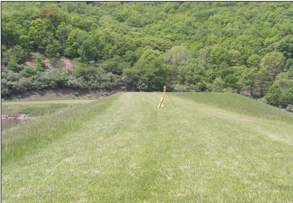
Figure 4 - Top of NC 14 (Propose to Raise Height with Concrete Parapet Wall).
