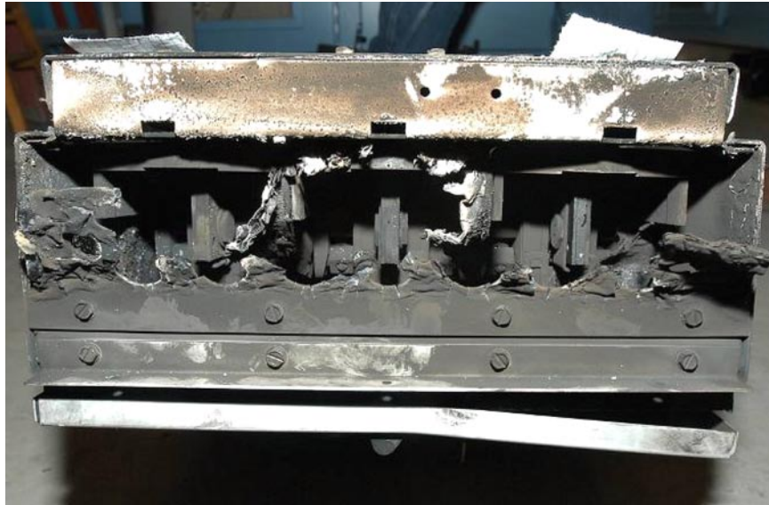
Figure 1-2. Bowed cover on switch 3A
