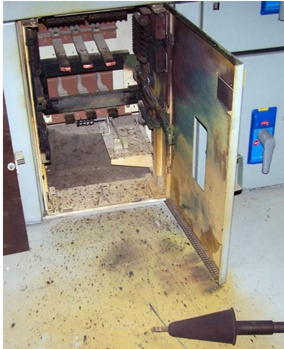
Figure 1-3. The damaged spare 480-volt circuit breaker cubicle and hot stick on scorched floor
