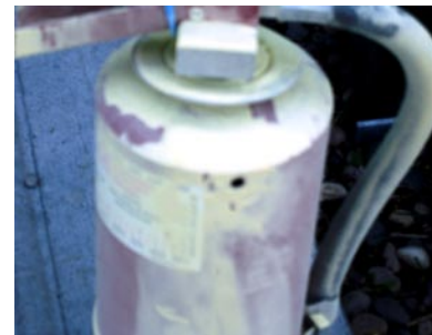
Figure 3-2. Hole in fire extinguisher
