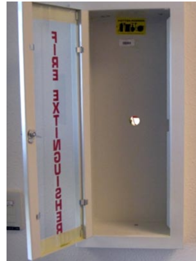
Figure 3-1. Hole drilled through back of fire extinguisher cabinet
