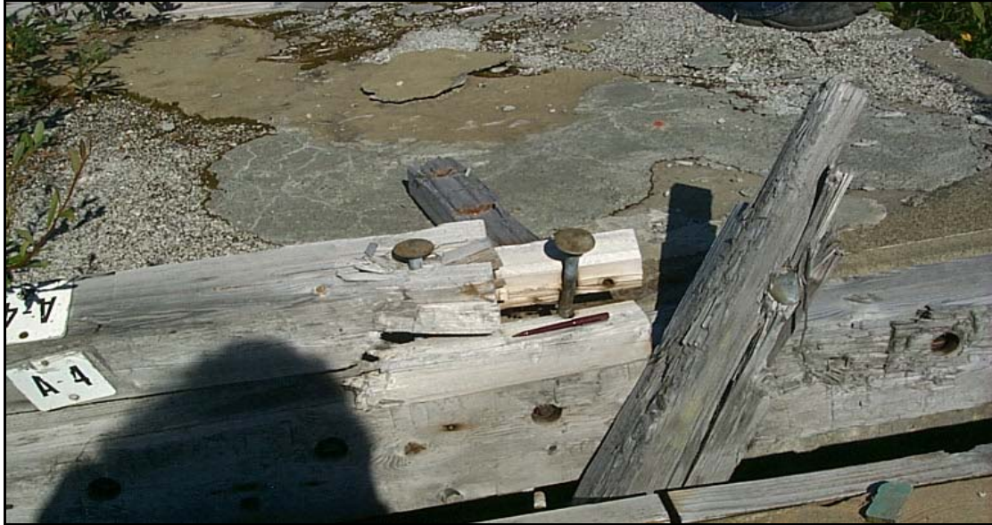
Figure B-3. Valdez Harbor Dock Damage Example
