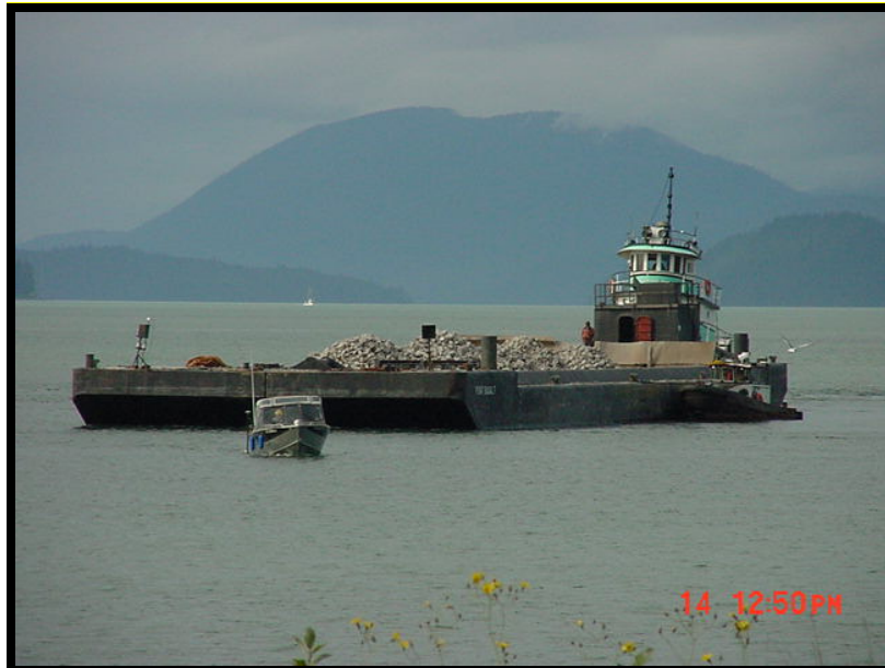
Photo 1. Split Hull scow with tug, positioning in preparation for core rock placement at Wrangell Harbor.
