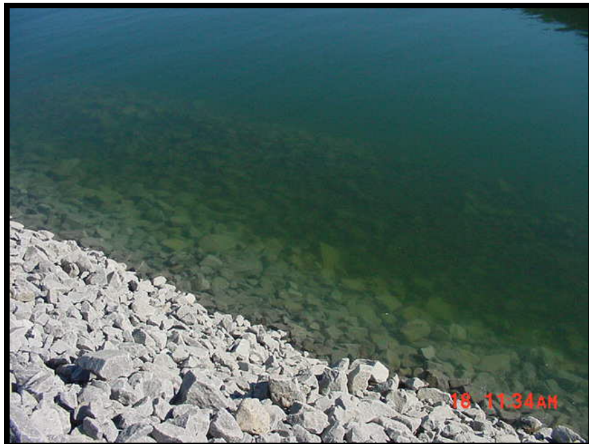
Photo 4. Core rock side slope projecting under water toward the toe at Wrangell Harbor.
