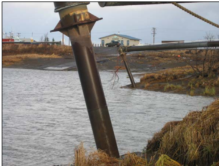
Figure 9: Damaged Swing Arms on East Bank of Dillingham Harbor West End study area
