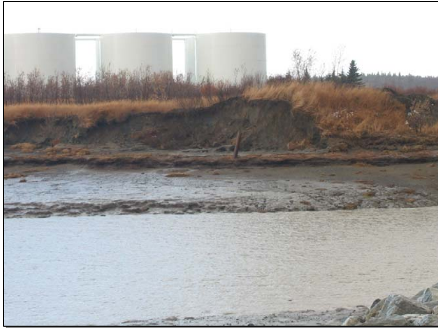
Figure 5: Erosion/Land Loss, West End Erosion Zone 1
