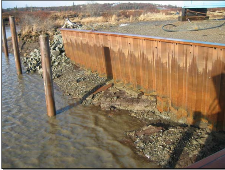
Figure 12: Erosion at West End of Harbor Bulkhead West End study area
