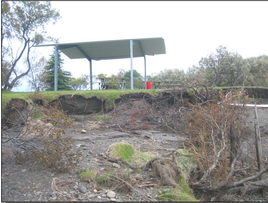
Figure 20: Erosion at Dillingham City Park looking West (September 2005)
