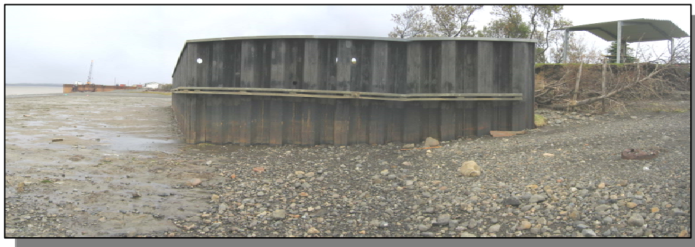
Figure 16: Erosion Outflanks West Terminus of Seawall – City Dock Side (September 2005)
