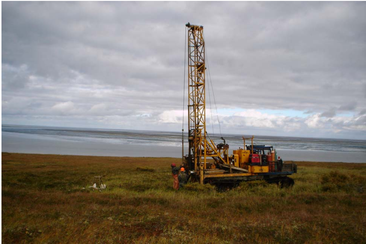
Photograph 1. Drilling operation at Test Boring AP-21 showing vegetation and topography of Mertarvik with the Ninglick River in the background.
