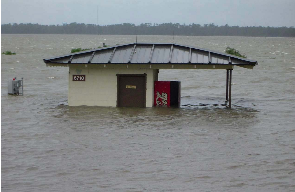
Hurricane Katrina's record low pressure, 125 mph winds and high tides converged to create a storm surge that raised the level of the Back Bay of Biloxi nearly 30 feet above normal. This restroom lies between the 12th and 13th holes on the Keesler AFB golf course (USAF photo).
