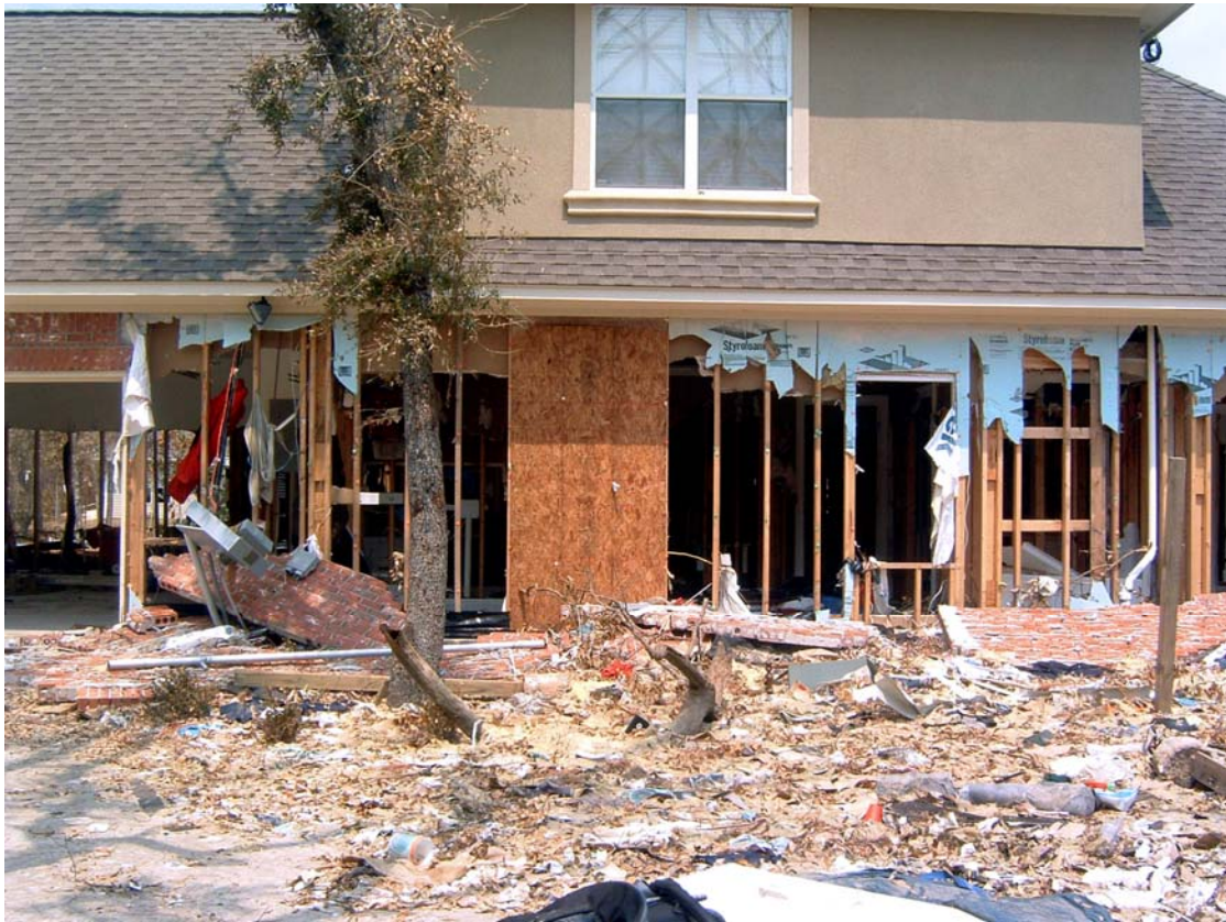
Hurricane Katrina ripped away brick and sheetrock from the first floor of SMSgt David Hufton's home in Ocean Springs, Mississippi, but left the second floor seemingly unscathed. He and his family had not even lived in the house for a month before it was destroyed by the hurricane. The intelligence analyst with the 403rd Wing at Keesler AFB, Mississippi, stayed with his family at a hotel near Dobbins Air Reserve Base, Georgia, after the storm (USAF photo by SMSgt David Hufton).
