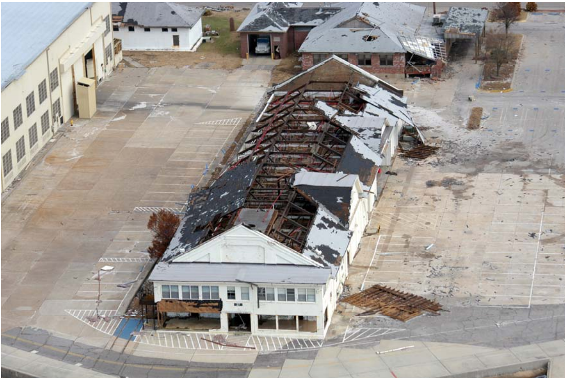
Building 27, Naval Air Station Pensacola Photo Lab, and the water survival equipment storage building, show considerable amounts of roof damage after Hurricane Ivan slammed into the base. Navy officials reported that nearly 90 percent of the buildings on the base suffered significant damage (U.S. Navy photo).
