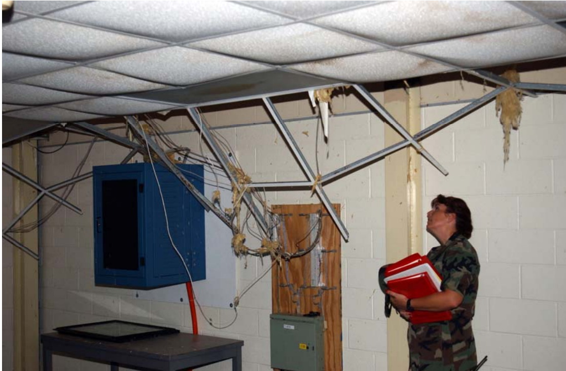
1st Lt Wendy Hendley, 403rd Wing facility manager, inspects damage for Air Force Reserve Command civil engineers during AFRC's assessment team visit to Keesler AFB, Mississippi, on 20 September 2005. Many of the command's office buildings, maintenance shops and hangars were severely damaged by Hurricane Katrina (USAF photo by Lt Col Bob Thompson).
