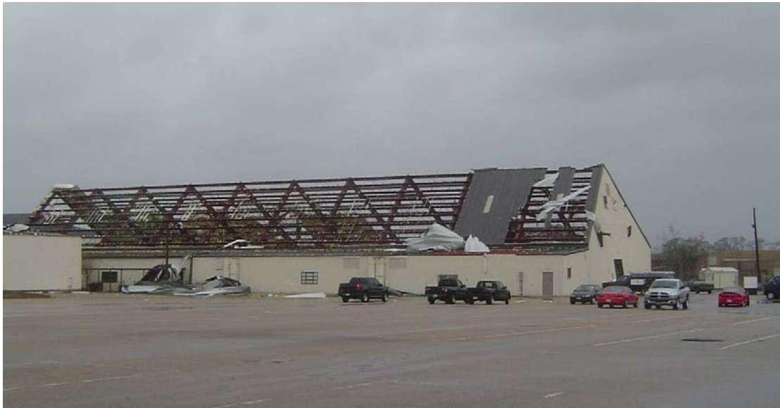
Winds gusting to 140 mph heavily damaged the older roofs on Keesler AFB. Newer construction fared better, because the more recent buildings had been designed to withstand Category 5 winds.
