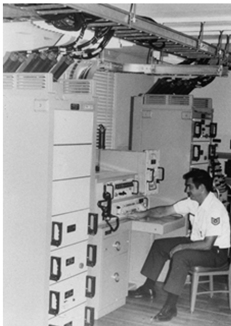
Shown is a view of communications equipment used with the Minuteman launch training facility.
