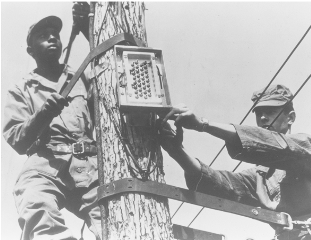
These student repairmen install a terminal box atop a telephone pole. This is an example of the practical training received in the installer repairman phase of the fixed wire communications course at Francis E. Warren AFB, Wyoming.
