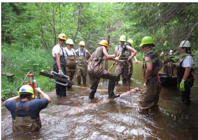
Volunteers installed logs in the river bed to provide improved stream flow and fish habitat.
