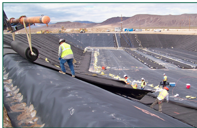
Workers install one layer of the liner system for the new Mixed Waste Disposal Unit at the Nevada National Security Site.
