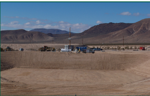
The RCRA-permitted Mixed Waste Disposal Unit is an excavated facility engineered with a leachate collection system and double-liner with multiple layers of geosynthetic clay, high-density polyethylene, netted fabric, and screened native soil.
