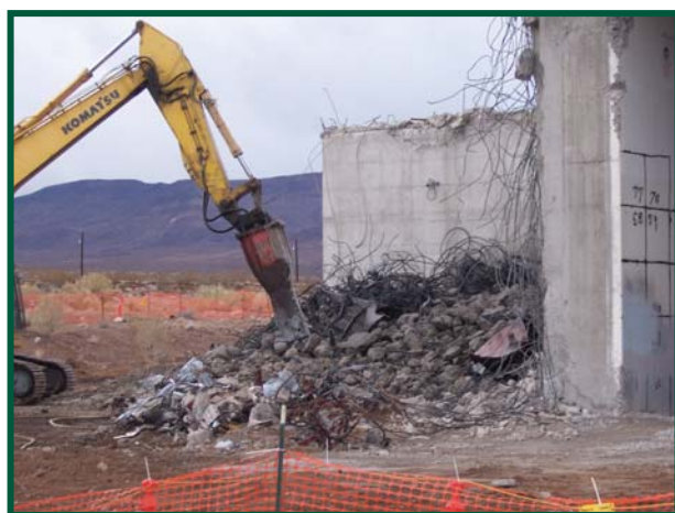
Demolition of the Reactor Maintenance, Assembly, and Disassembly decontamination building at the Nevada National Security Site.
