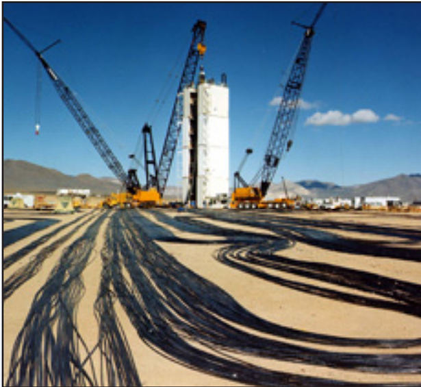
A temporary modular tower designed to hold the diagnostic rack for Icecap is a current landmark at the Nevada National Security Site.
