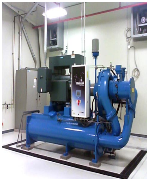
FIGURE 2. 1,500 hp centrifugal compressor system
