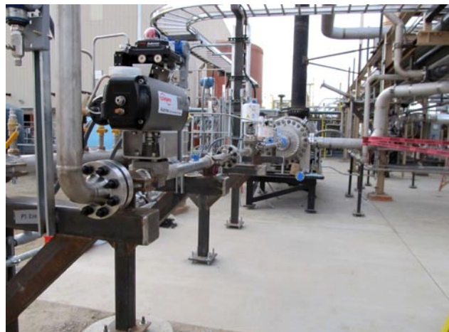
FIGURE 4. RH test rig installed at CES Kimberlina
