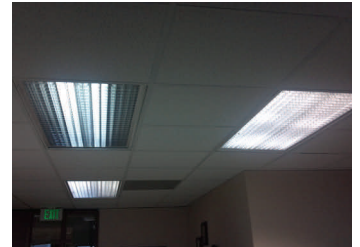
The left near fixture is emergency lighting that is lit continuously. Two LED tubes replaced four fluorescent tubes, providing long-term energy savings.
