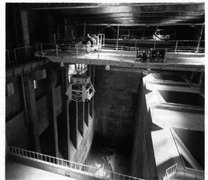
Refuse Pit and Crane
