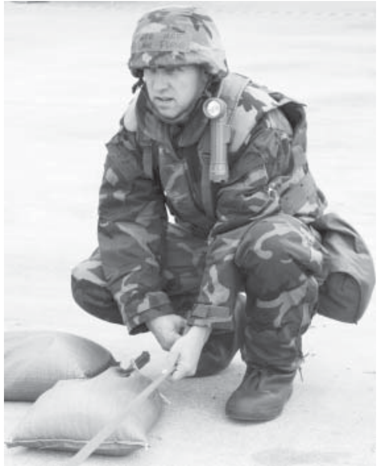
Major Flolo measures off distance for a wall of a bunker built from sandbags during hands-on training. (U.S. Air Force photo by Tech. Sgt. David D. Morton)
