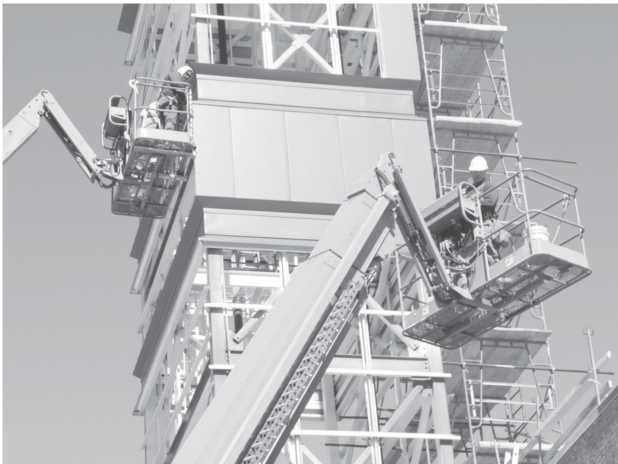
Arturo Quintana, Terry Bopp and Luis Esquirel, roofing laborers, Central State Roofing Co., work from high-rise platforms on the parachute tower during construction of the new 39th Aerial Port Squadron and 302nd Airlift Control Flight facility. (U.S. Air Force photo by Tech. Sgt. David D. Morton)
