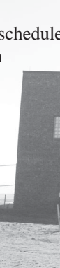
The new consolidated aerial facility is under construction. (U.S. Air Force photo by Tech. Sgt. David D. Morton)
