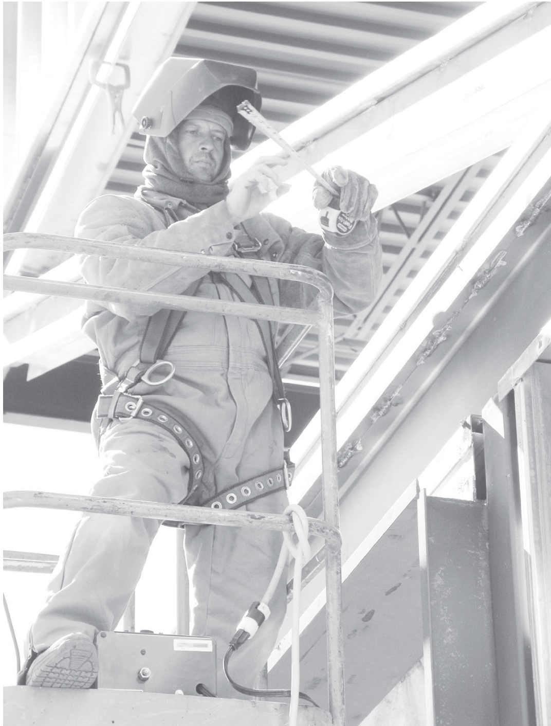
Bruce Edwards, carpenter, John Bowman, Inc., prepares to measure a framing beam during construction on the corrosion facility in March. (U.S. Air Force photo by Tech. Sgt. David D. Morton)
