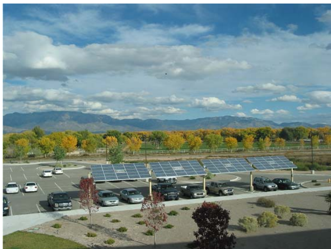
Figure 2. Large PV 6.kW Array.
