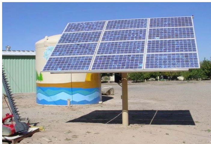
Figure 3. Polycrystalline 1.2 kW PV water pumping system with active tracker, and 10,000 gallon storage tank located at SIPI greenhouse complex. Pumps water for the arboretum, garden, and fruit orchard.
