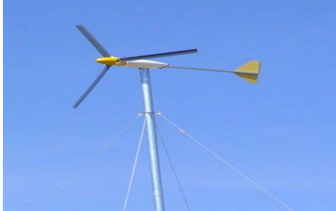
Figure 1. Bergey wind turbine installed at SIPI greenhouse complex.
