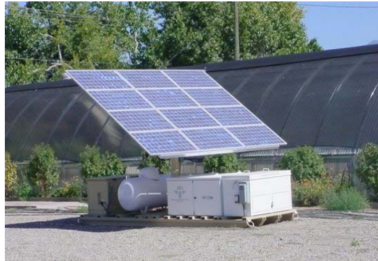
Figure 4. Stand-alone hybrid PV system for rural domestic electrification.
