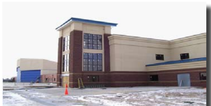
South entry, Squadron Operations Facility. Corrosion Control Hangar in the background
