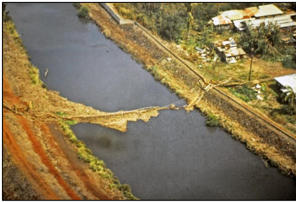
Stream Access Flooding Damage (Iniki)
