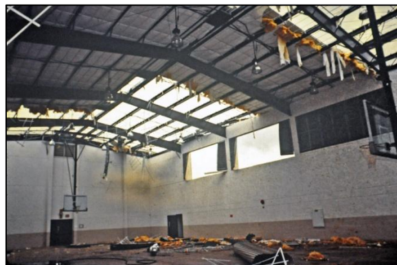
Roof Damage to Hanapepe Armory (Iniki)
