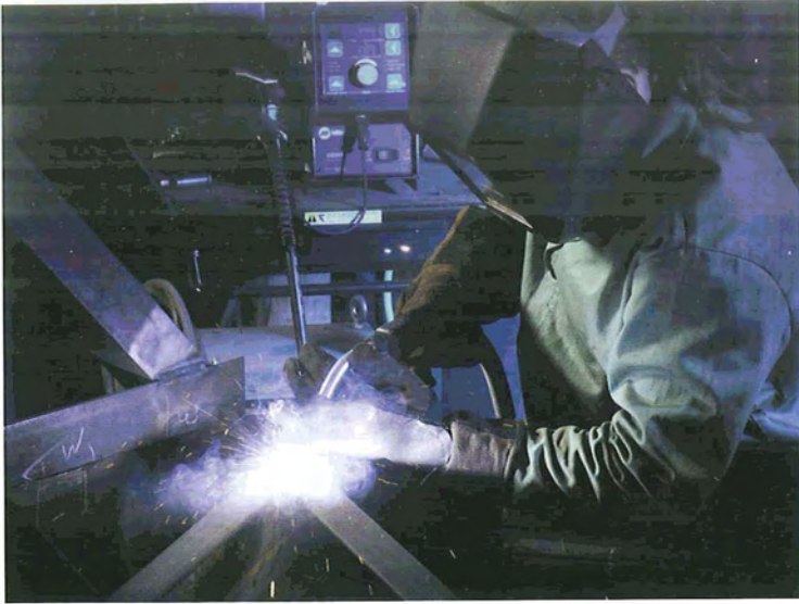
Bob Peters, of Kendel Welding and Fabrication, welds part of an internal access support for the Ares I-X upper stage simulator at NASA's Glenn Research Center in Cleveland. In 2009, NASA will launch Ares I-X, a test flight for the new Ares I rocket. Ares I will launch astronauts on missions to the space station, the moon and beyond. (21995main_image-eng)
