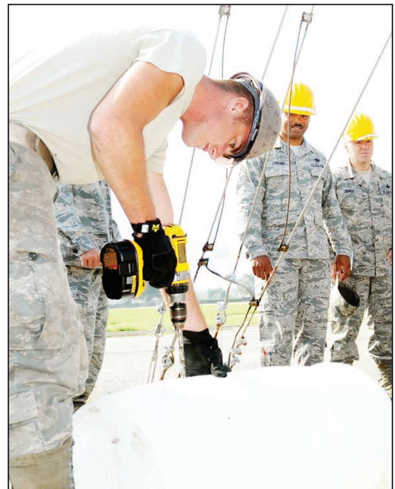
Airman 1 st Class Joshua Bogenrief, 85 th EIS, drills holes in a plastic barrel to be used in an underground trench.
