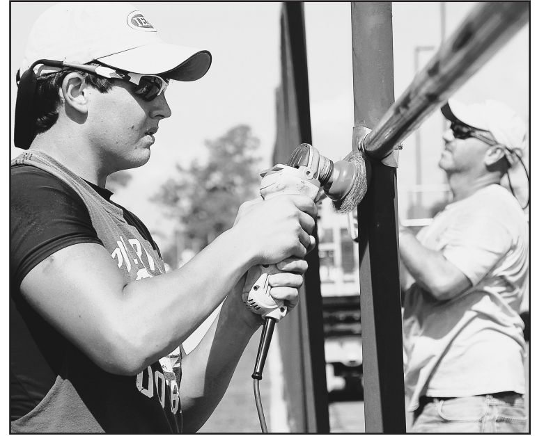
Photo by Kemberly Groue Laborer Zack Bates, left, and project supervisor Billy Spiers from Industrial Environmental Management of Poplarville, Miss., sand the poles surrounding the tennis courts on Meadows Drive for repainting July 19.
