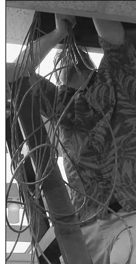
Billy Smith, 81st TRSS, prepares network cables for the new server rack at Vandenberg.
