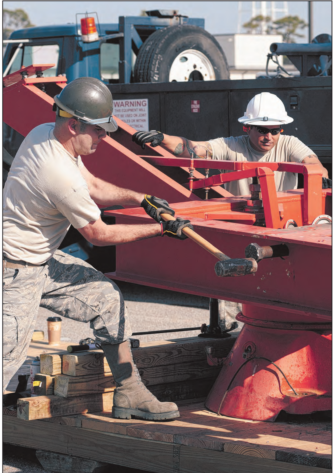
Staff Sgt. Steven Flint, left, 85th EIS, hammers out a retaining pin in the antenna pedestal as the team chief, Tech Sgt. Walt Ferrell, observes other Airmen perform the finishing touches on the radar dismantling.
