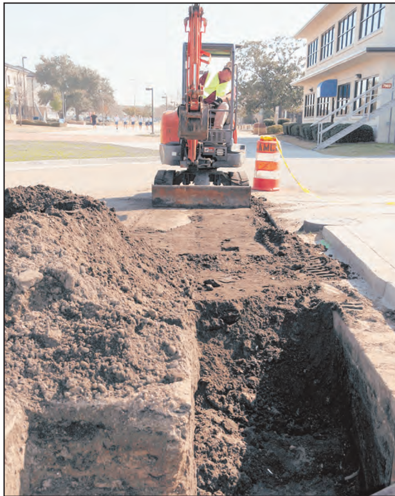
Dennis Mason from Shackleford Plumbing prepares a ditch for pipe-fitting for the Triangle’s chilled water loop project in front of Triangle Fitness Center, Feb. 15.
