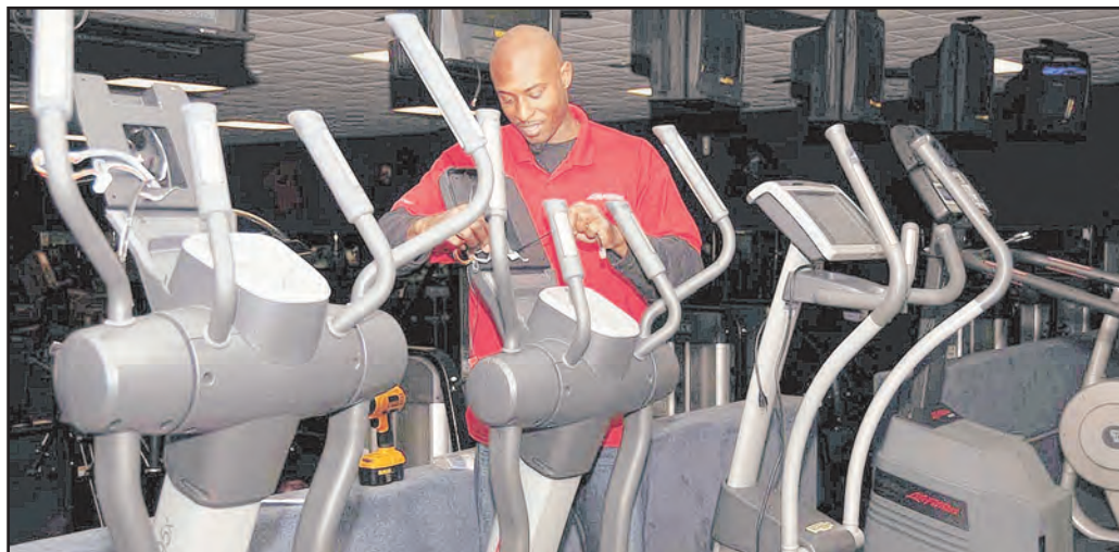
Installer Kenneth Jackson from Life Fitness, Atlanta, assembles a line of elliptical equipment Friday at Triangle Fitness Center.
