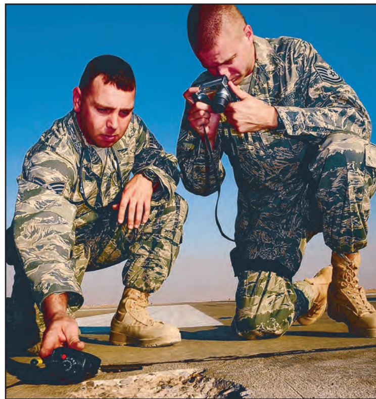
Photo by Tech. Sgt. Johnny Saldivar Sergeants Hughes, left, and Gross photograph damage to a runway.
