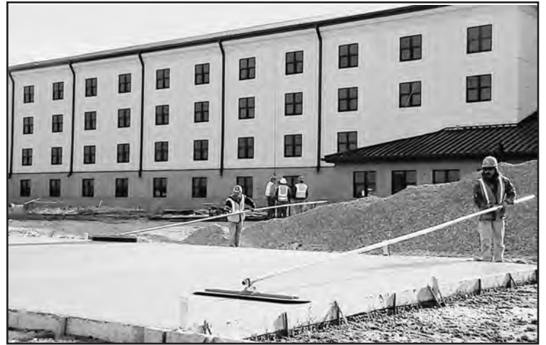
Roberto Frias and Victor Mejorado from Valley Crest trowel the troop walk outside the new dorm.
