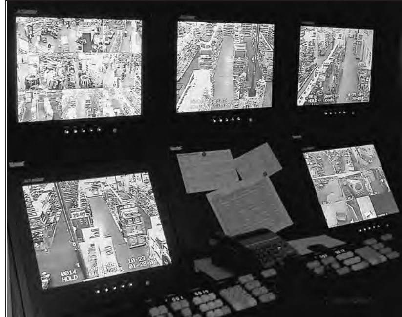
Surveillance cameras at the main exchange allow AAFES personnel to monitor activity throughout the facility.
