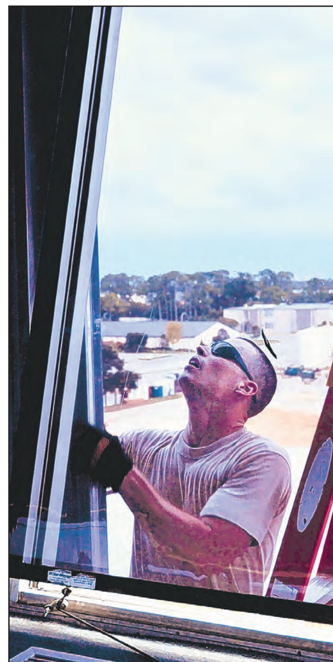
Photo by Adam Bond Staff Sgt. Matthew Osborn, 81st CES, hardens the air traffic control tower windows prior to Gustav's arrival.
