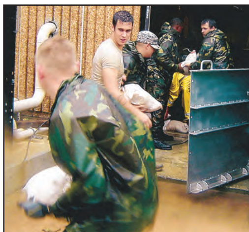
81st Civil Engineer Squadron photo Members of the 81st CES form a sandbag brigade to protect Keesler Medical Center.
