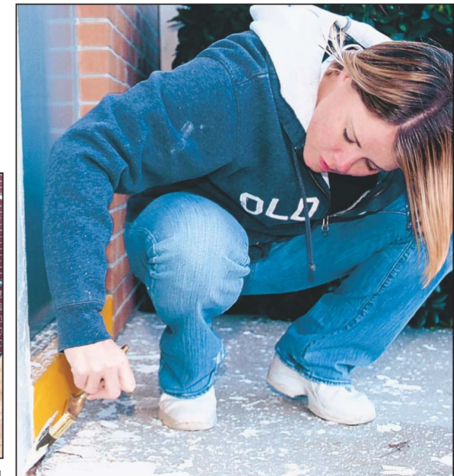
Photo by Adam Bond Staff Sgt. Cassandra Key, 81st Medical Group, touches up the paint job on support columns at Jeff Davis Elementary School in Biloxi. Keesler had more than 400 people involved in 35 projects all along the Mississippi Gulf Coast.
