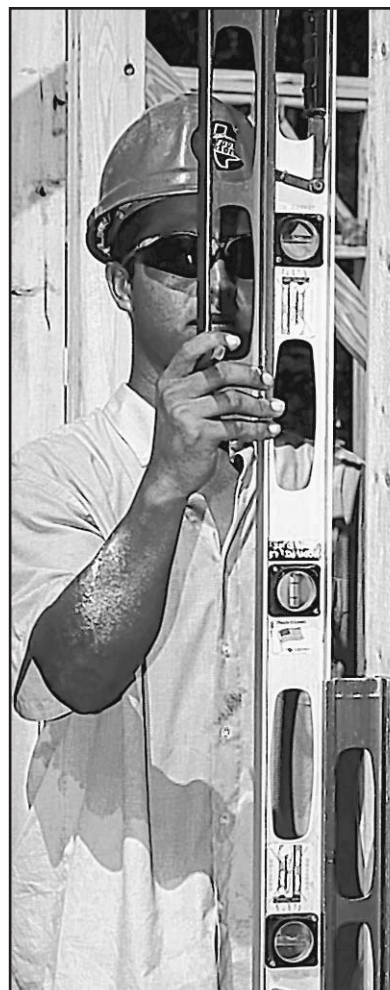
Diego Alvarez plumbs the interior walls in the first framed house in Thrower Park.
